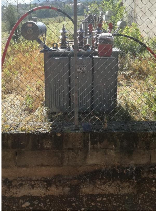
Figure 61. Three-phase step-down transformer supplying the cable-joint system.
