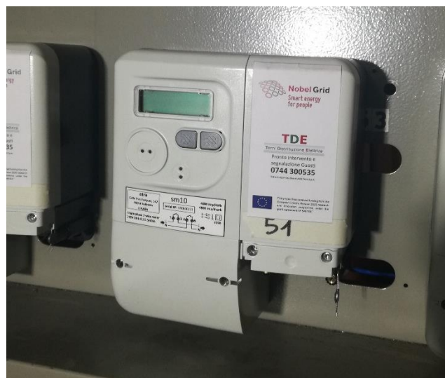
Figure 96. SLAM installation in an apartment building (details)
