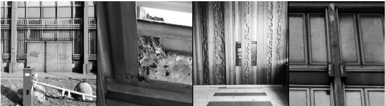
Fig. 4 Elements of detail degradation of the building: the outdoor area, an aluminium frame, the boiserie in the entrance hall, the curtain wall.
