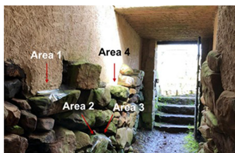
Fig. 1. The red arrows mark the specific areas in the underground environment where the HVPD formulations were applied.
