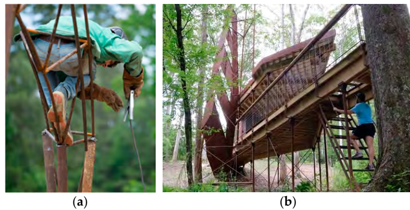
Figure 10. (a) Self-construction and “low-tech” student preparing to weld the shade structure of the Pisces Bridge. Photo credit Michael Tolar. (b) PEREGRINE zip line student demonstrating the tree house floor hatch. Photo credit, Brad Deal.
