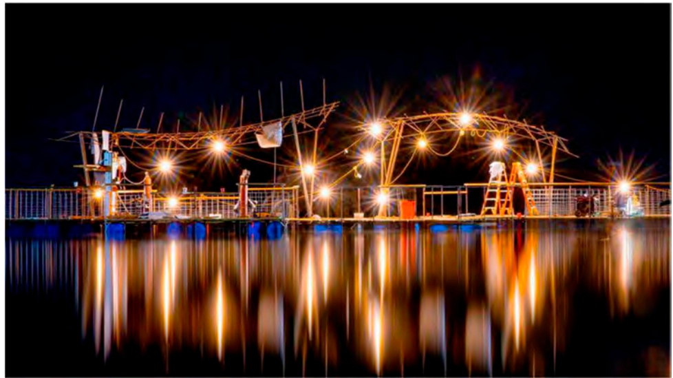
Figure 6. PISCES BRIDGE on its final night of construction. Photo credit: Brad Deal.
