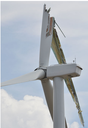
Figure 1.5: Structural failure of a wind turbine at Invenenergy’s Prairie Breeze wind farm.
