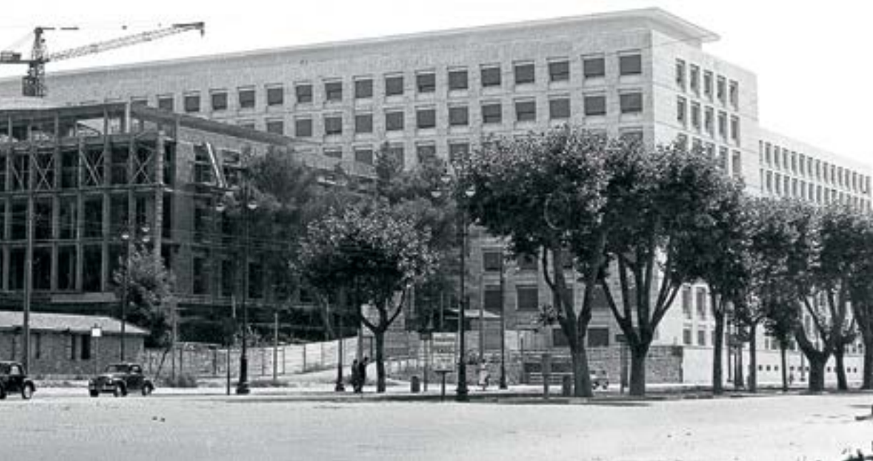
On the opposite page: The site from above during construction of building A. Top left: The FAO complex during construction of building A.
