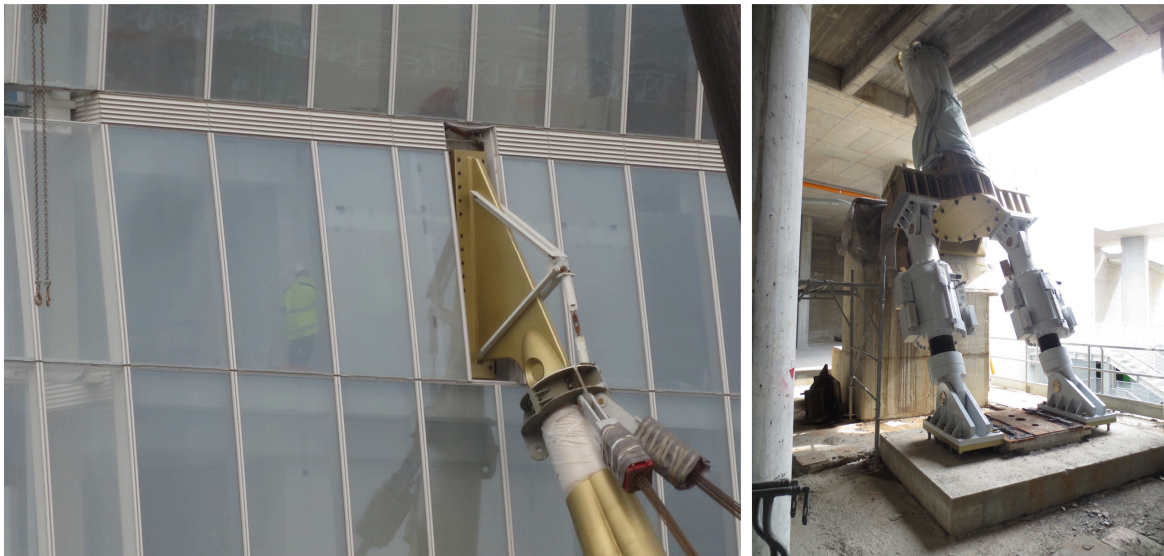
Figure 7.5: Detail of the strut connected at the top to the curved glazed façade and constrained at the base to a pair of viscous dampers
