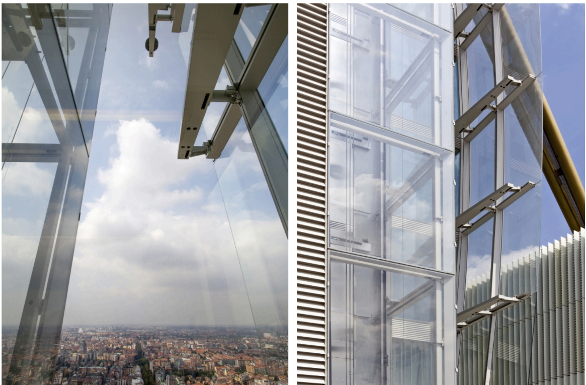
Figure 7.9: Detail of the curved glass cantilevered at the extremity of the façade. Source: https://www.focchi.it/it/
