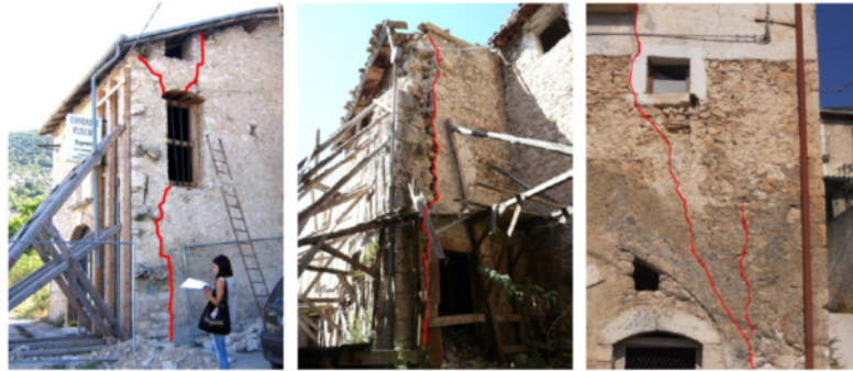
Figure 16: Observed building damage mechanisms, San Pio delle Camere.
