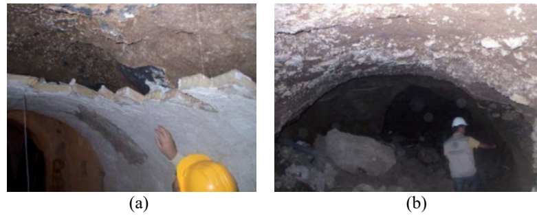
Figure 10: Qualitative survey of the hypogeal structures: assessment of the structural status (a); material and humidity level (b). The first team analysed the main structural characteristics of these chambers, such as the soil type and the humidity level (Figure 10a, b). Clay alluvium of red colour was mainly identified, with discrete cohesion and compact. Due to the lack of instrumentation, the survey was performed in qualitative but systematic way, which is sufficient for general information. The students could associate the chamber qualitative features to their structural behaviour: their stability is due to some low tensile material strength and plastic behaviour.
