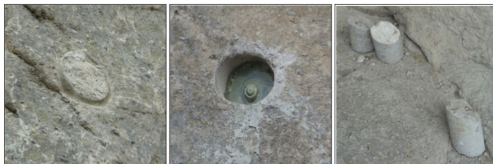
Figure 8. Rock core drilled used for mitigation (left), bar insertion (center) and bolt sealing (right).
