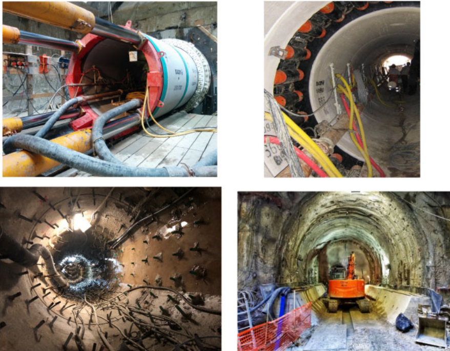
Figure 4. Mini-TBM at the launching pit and at the intermediate jacking station (a-b); mini tunnel at the completion of radial injections (c); conventional tunnelling in the improved soil.
