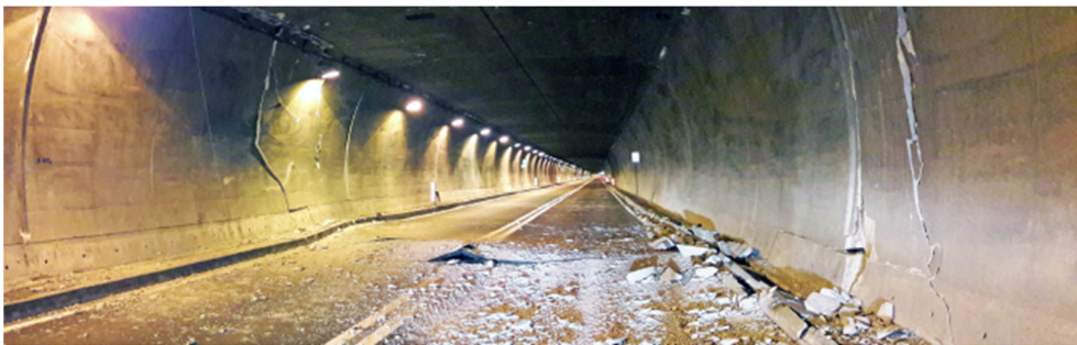
Figure 3: Damage to the concrete segments and the pavement of the San Benedetto tunnel due to the Norcia earthquake.
