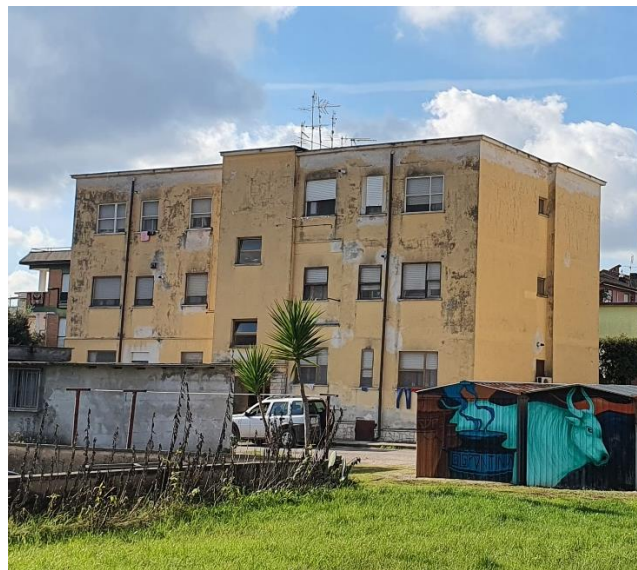
Figure (01-54) An example of a rural building by construction condition Pontinia, Lazio Region (taken by the author).
