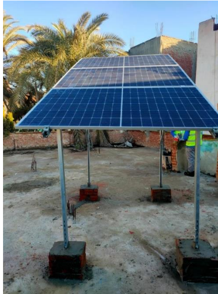
Figure (04-22) The solar plant after installation resulted from implementing the Scrum framework.
