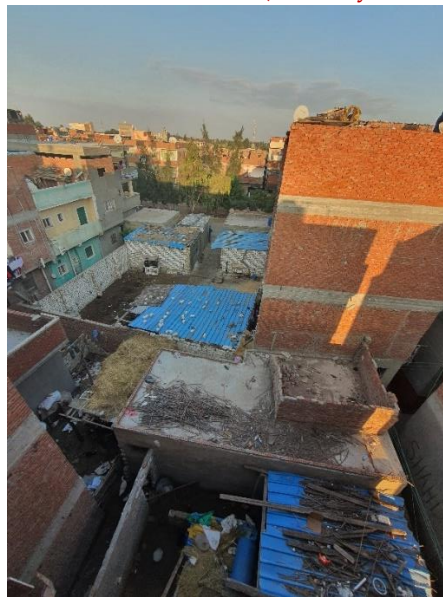
Figure (01-94) Typical in-between space configurations, used as poultry and bird farms and stores. The light structure consists of red brick walls and corrugated galvanized steel sheets (taken by the author).
