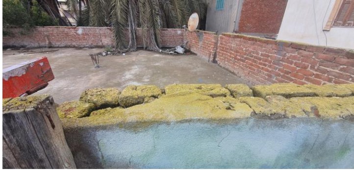
Figure (04-20) Green molds fungus indicates that the client ignores the roof, reflecting the maintenance behavior towards the solar plant. (taken by the author).
