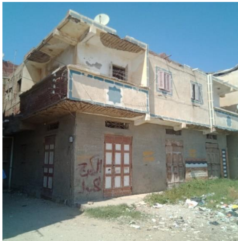
Fig (01-48) A dwelling in a rural settlement in a bad construction condition and requires significant rehabilitation (taken by the author).
