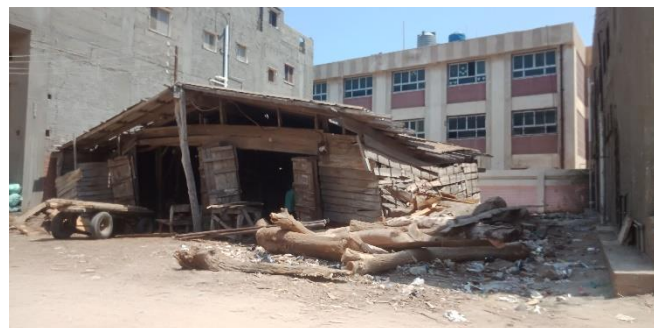
Figure (00-05) A warehouse shows fishing culture's Impact on the built environment in a traditional coastal settlement in Egypt (image taken by the author).
