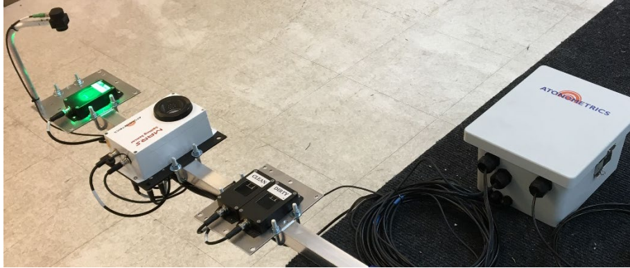
Fig. 2 Atonometrics equipment for testing DUSST side-by-side with a reference cell pair as well as the MARS sensor.
