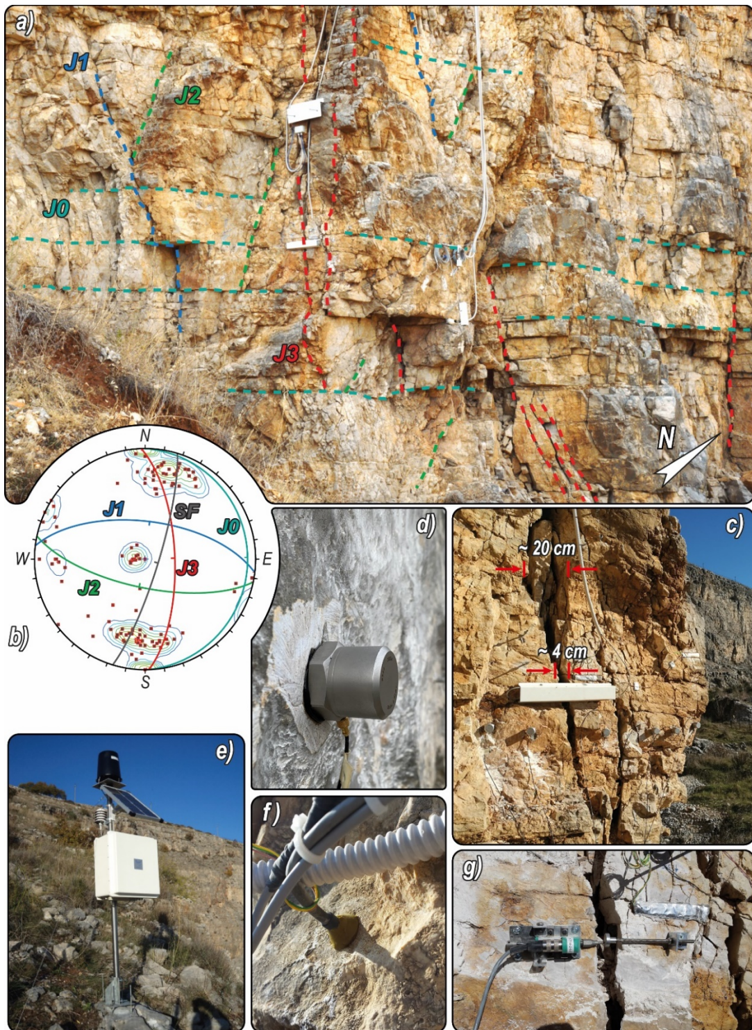
Figure 3.13. Representation of the main joint traces dissecting the monitored rock block and the adjacent quarry wall sector (a); Synthetic stereographic projection (equal-angle lower hemisphere) representing pole density distributions and planes of the four main discontinuity sets, along with the direction of the slope face (SF) (b); open joint acting as the release system that separates the rock block from the rock mass (c); monoaxial microaccelerometer installed on the rock block surface during one of the performed long-term microseismic monitoring campaigns (d); fully-equipped weather station (e); temperature probe (f); extensometer installed on an open fracture along with a strain gauge placed on a microcrack and covered with aluminum tape for thermal insulation (g).
