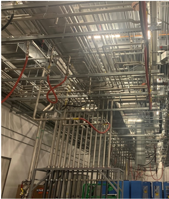
Figure 6: Klystron gallery installed cooling systems.
