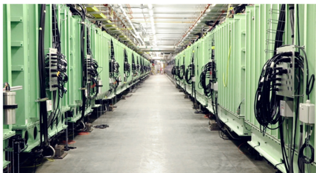
Figure 2: FRIB tunnel after the completion of installation.
