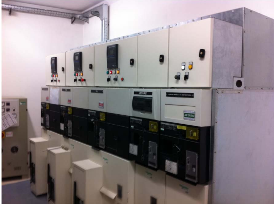
Figure 2. A MV Switchboard constituted by 5 units: for network supply, transformer, reserve, measures and tie switch
