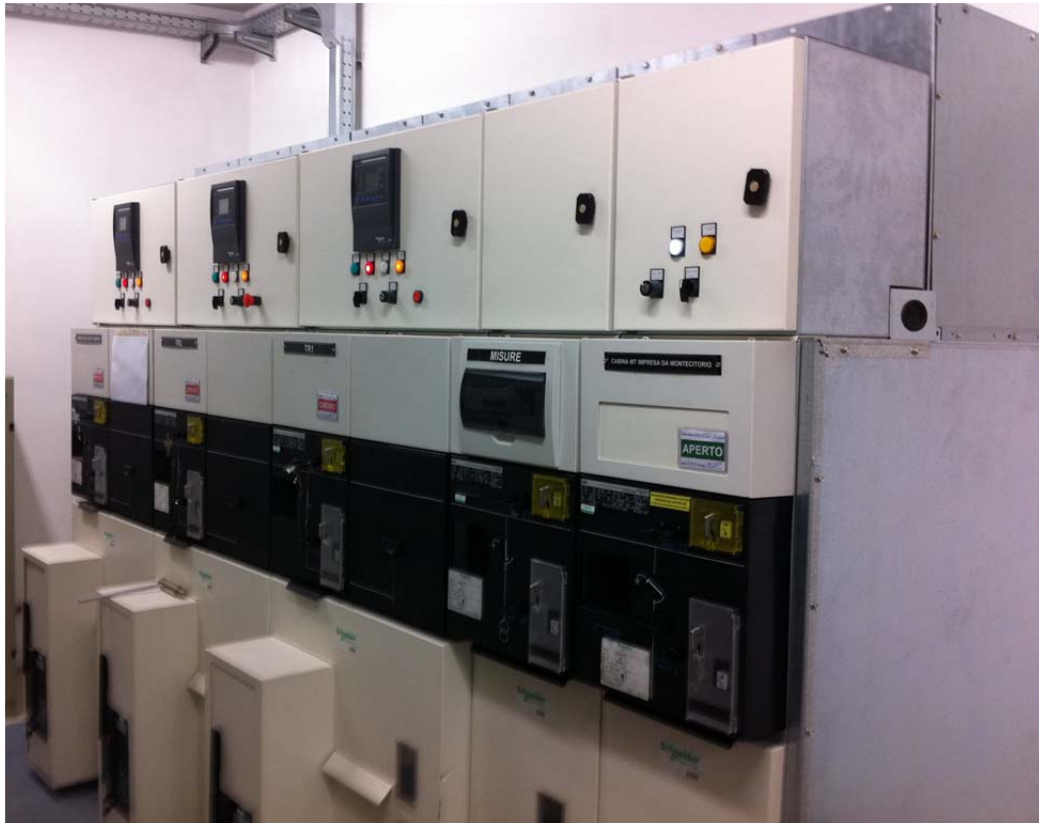
Figure 8. A MV SB of a transformer substation: a case of SB in two sections. The section is constituted by 3 CB-BI units, 1 MU and 1 IS unit as tie switch interconnected to the other SB section
