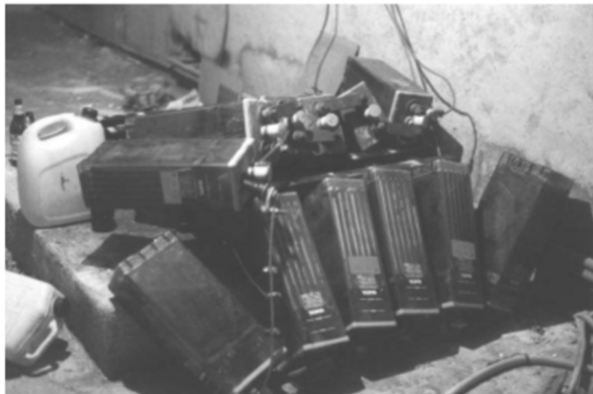
Figure 1. Batteries of an emergency generator set broken after an earthquake: the electrical service is not available because it is not possible
