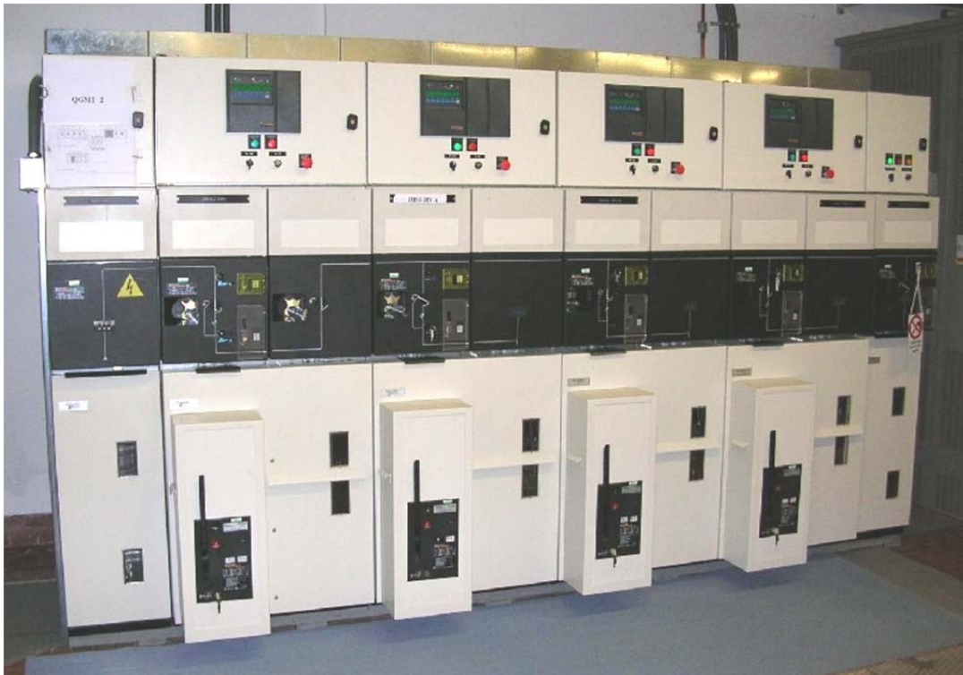
Figure 7. A section of the MV MSB: it is constituted by 6 units in particular 1 BR unit, 1 CB-DBI (for incoming utility), 3 CB-BI and 1 MU
