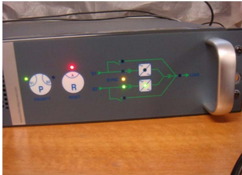
Figure 17. Warning signal given by the STS display: the transfer cannot be operated because the sources are not synchronized and characterized by a high phase shift
