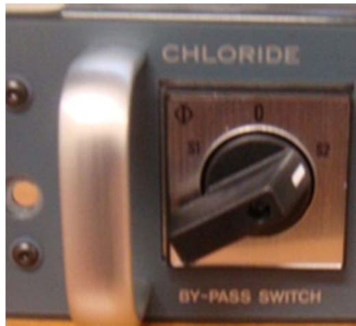
Figure 15. The manual STS by-pass switch
