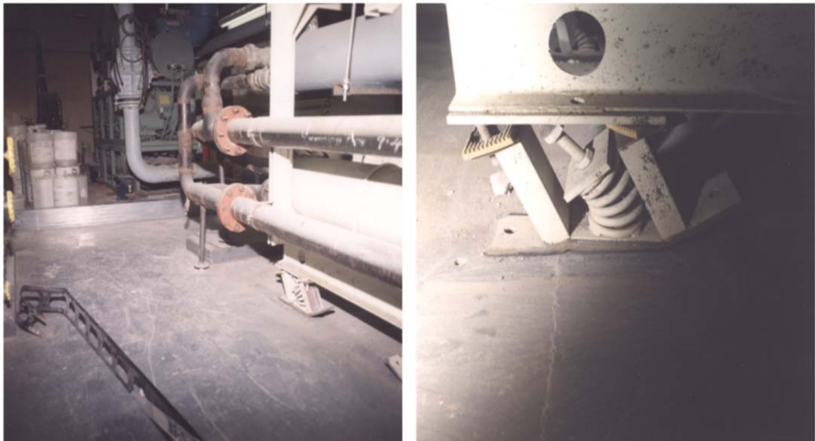
Figure 3. The support of a generator has collapsed after an earthquake. The emergency supply is not available
