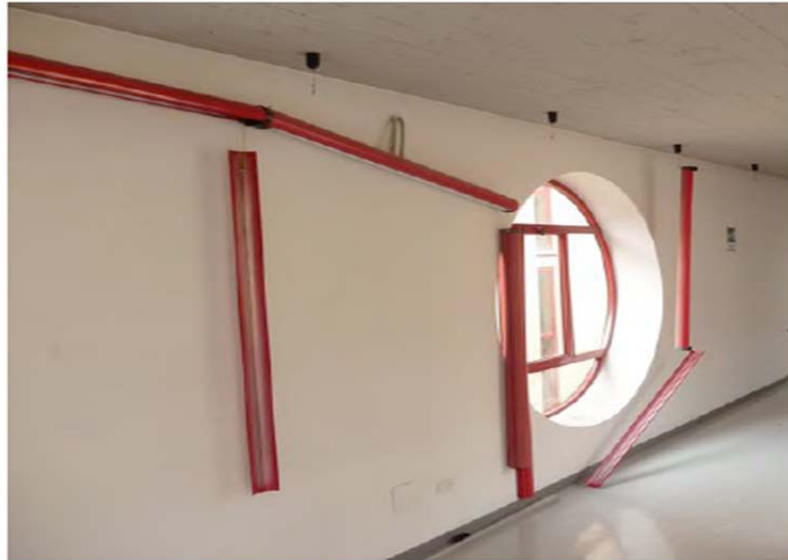
Figure 2. Lighting system damaged after an earthquake
