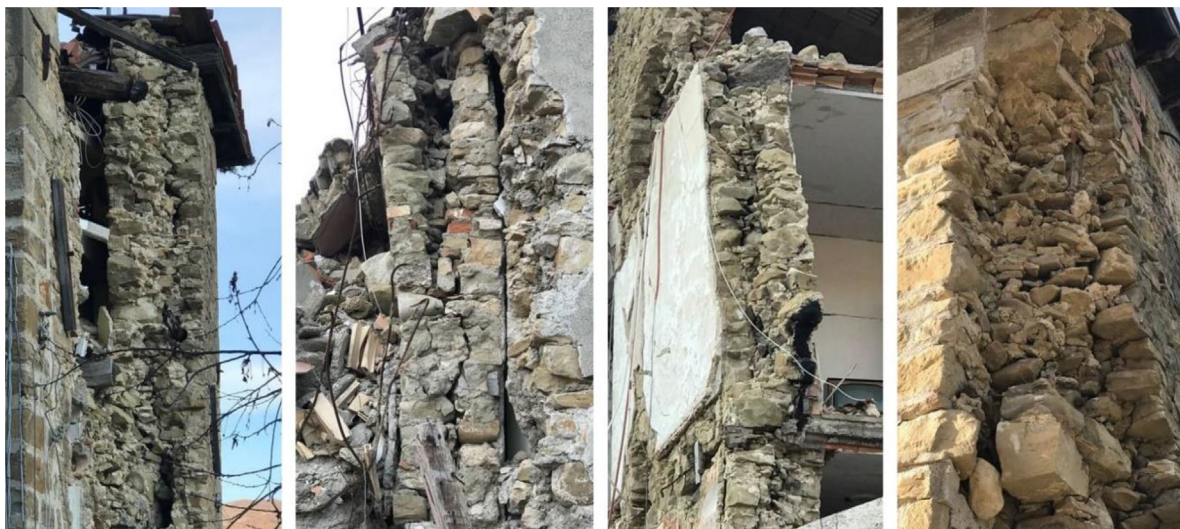
FIGURE 1 Wall sections and seismic damage after the 2016 Central Italy sequence
