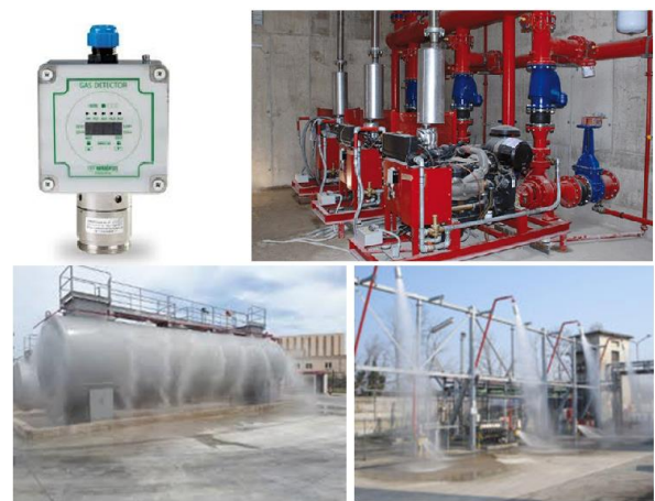
Figure 13. Safety measures for LNG plants: at the top left a gas detector, right, pumps of a fire-fighting system, bottom left and right systems for cooling tanks and loading area
