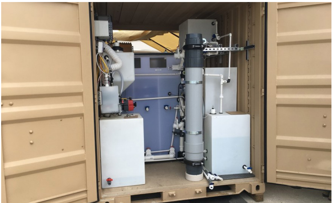
Figura 106: NEW generator USF
