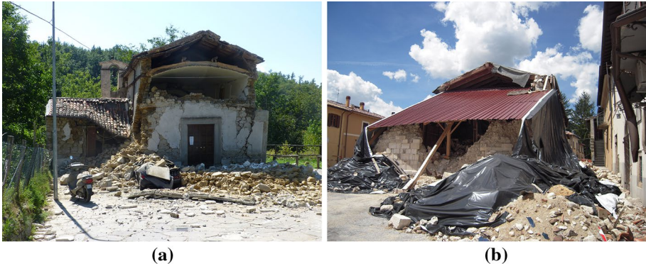
Fig. 8 Examples of poor masonry quality causing wall disintegration: a San Lorenzo Martire, Cossito (Amatrice); b Santa Rita, Norcia
