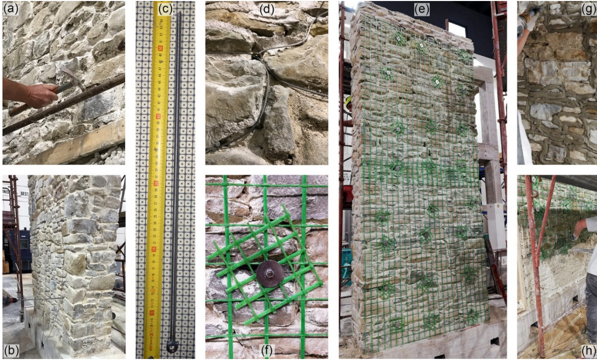
Figure 5. Phases of the strengthening works on CR wall: removal of the mortar from the joints of the external side (a); drilling of the holes for the connectors (b); stainless steel connector (c); stainless steel cords placed in the mortar joints (d); GFRP mesh laid over the internal side (e); nut-washer-patch at connector-mesh intersection (f); repointing of the mortar joints of the external side (g); machine application of the thermo-insulating mortar over the GFRP mesh of the internal side (h).
