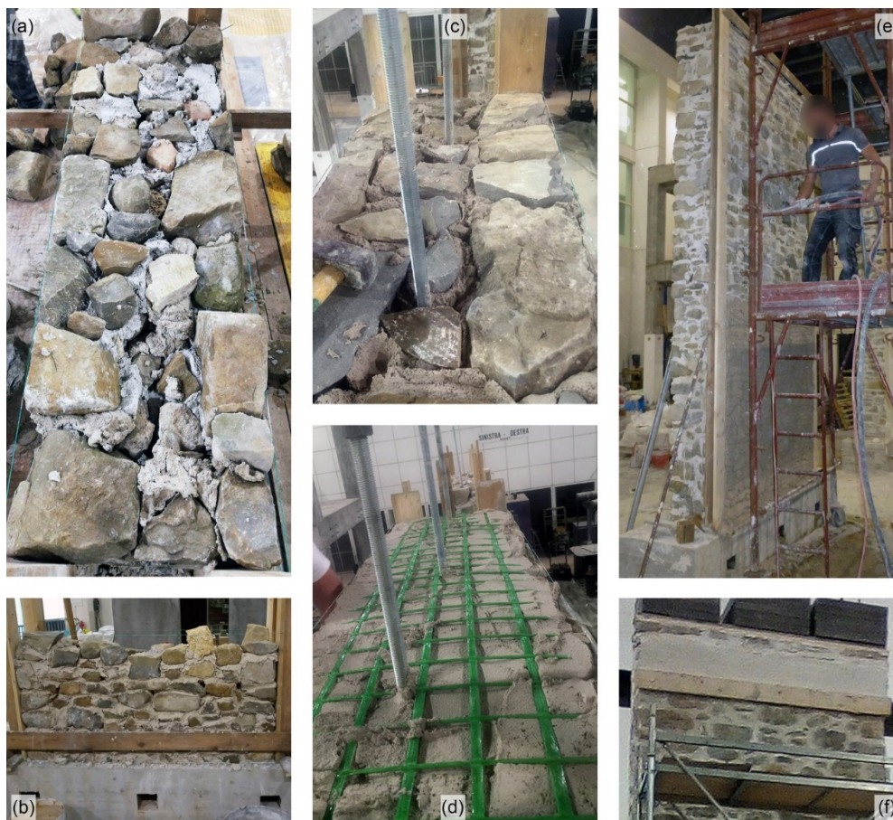
Figure 1. Construction phases and details of the wall specimens: horizontal stonework layer (a), elevation of the fair faced side (b); top vertical connectors (c); reinforced masonry top beam (d); machine application of the plaster layer on the internal side (e), plaster band on the crowning beam (f). Pictures referred to CC wall.
