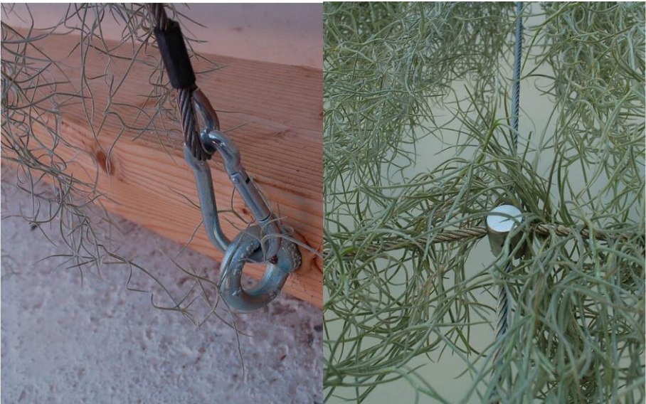
Figure 2. Left: detail of the anchoring system of stretched cables to the ground through a wooden beam; right, detail of the steel mesh knots.
