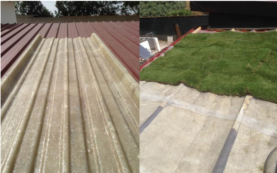
Figure 3. Left: installation of the trays on the roof for the experimentation phase; right, detail of the installation of the cultivation layer
