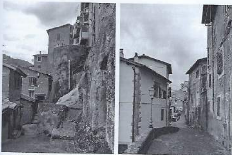
Figures 14–15. Modern transformations in the historical buildings of Genazzano (Roma). On the one hand, the replacement of coverings, hindering the direct survey of the fabrics, rather alters the perception of the state of conservation, making it falsely good. On the other hand, the addition of balconies, revealing horizontal overlapping among different building systems, worsens the index of vulnerability
