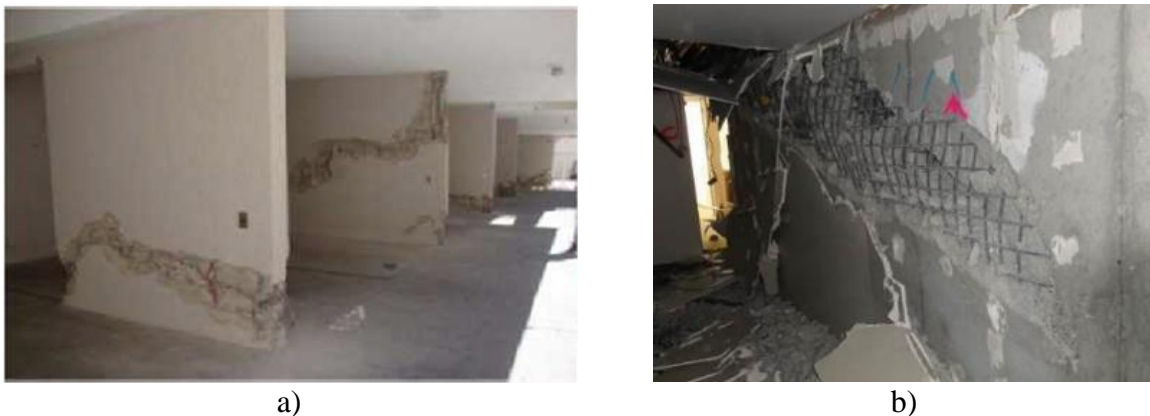
Figure 1: Observed damage to RC structural walls in a) the 2010 Chile earthquake [3] and b) the 2011 Lyttleton earthquake, New Zealand [2].
