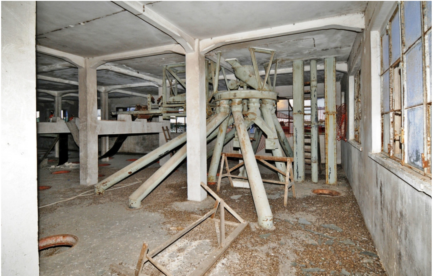
One of the rotating distributor units for filling cells in the Silos, with the characteristic Hennebique reinforced concrete structure.
