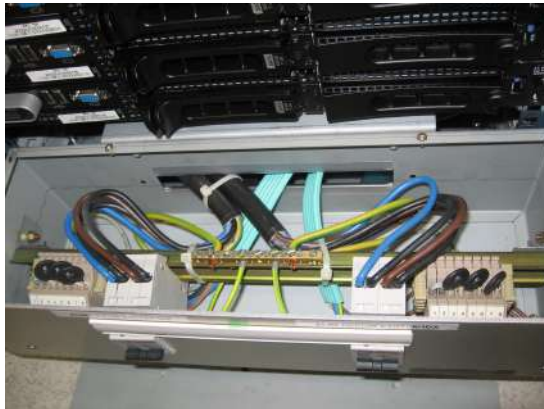
Figure 64. View of the interior of a repartition box.
