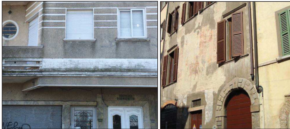
Figure 2.39. Damage to non-structural components due to material obsolescence (source: www.infobuild.it ).
