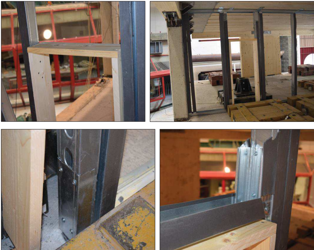
Figure D.3. Partition in the wall direction: timber frame forming a door in the partition wall (top - left and right); detail of the connection of the steel studs forming the openings to the bottom horizontal profile (bottom - left); steel assembly above the timber frame (bottom - right).
