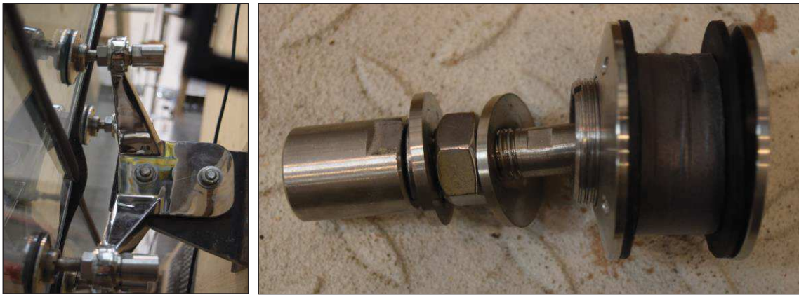
Figure 7.40. Misalignment of the spider connector (left) and one of the rotules elongated during the tests (right).
