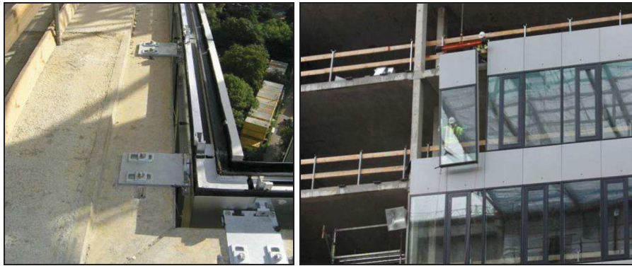
Figure 2.4. Unitised curtain system: example of connection detail and installation of the façade (source: www.archiexpo.com ).
