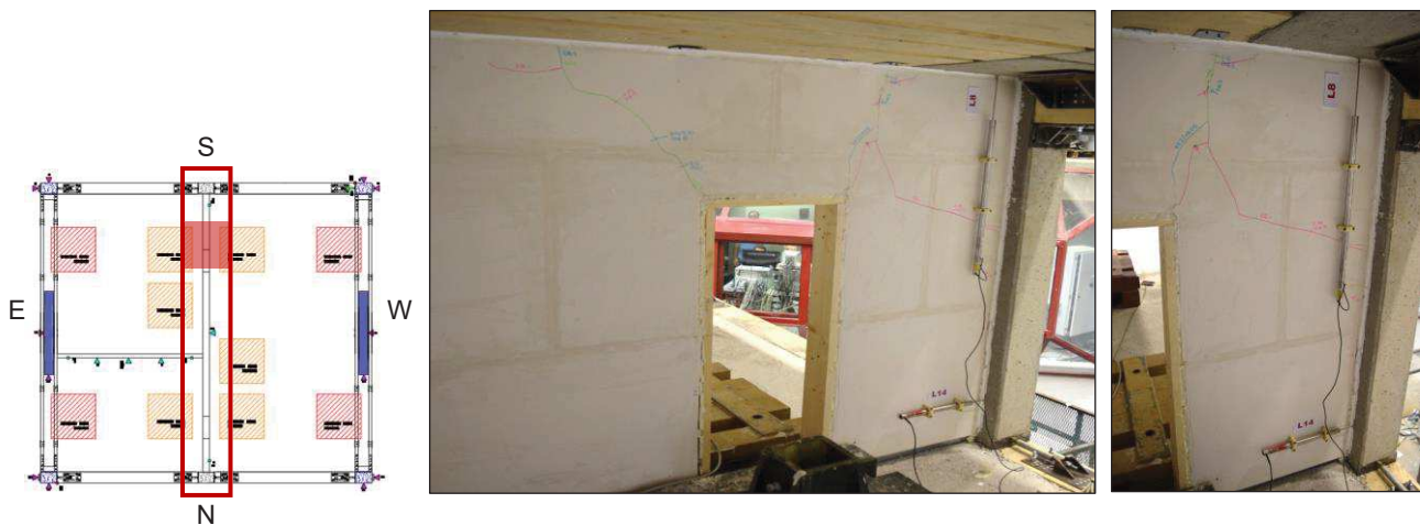
Figure 7.27. Cracking of the South-North wall in the East side, South opening.
