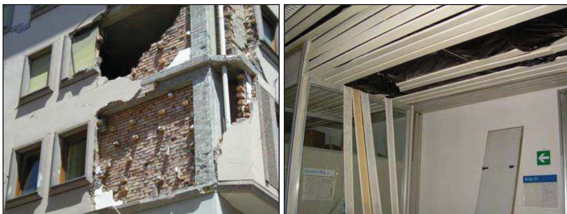
Figure 2.35. Damage to non-structural components due to earthquakes (De Sortis et al. 2009).
