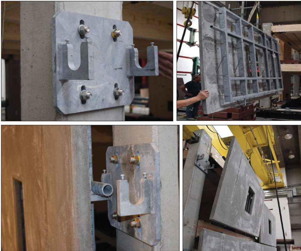
Figure 6.36. Assembly of the precast concrete claddings: connection of the upper anchorage to the concrete columns (top - left), lifting of the panels (top - right), particular of the sliding anchorage (bottom - left), positioning of the last panel forming the façade (bottom - right).
