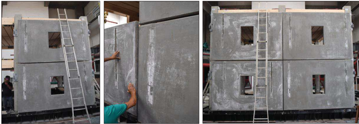
Figure D.12. Completion of the façade in the North side of the Test Building: assembly of the panels in the West part (left); lifting in place of the bottom panel in the East side (centre); final configuration of the façade (right).
