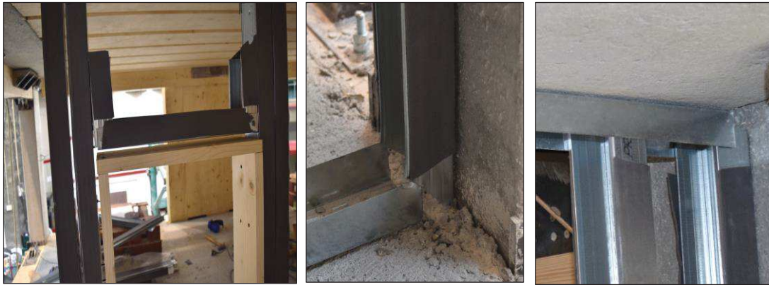
Figure 6.31. Steel frame construction: timber frame of the door opening with the upper steel assembly (left); lateral gap between the horizontal guide and the concrete column (centre); gaps on the top between horizontal guide and column as well as between vertical guide and horizontal profile (right).
