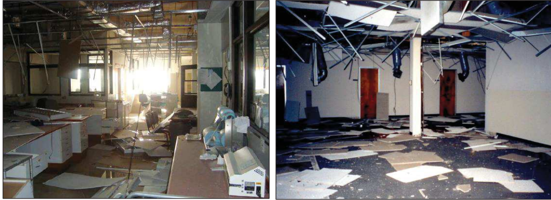
Figure 3.7. Damage to suspended ceilings (FEMA E-74 2011).
