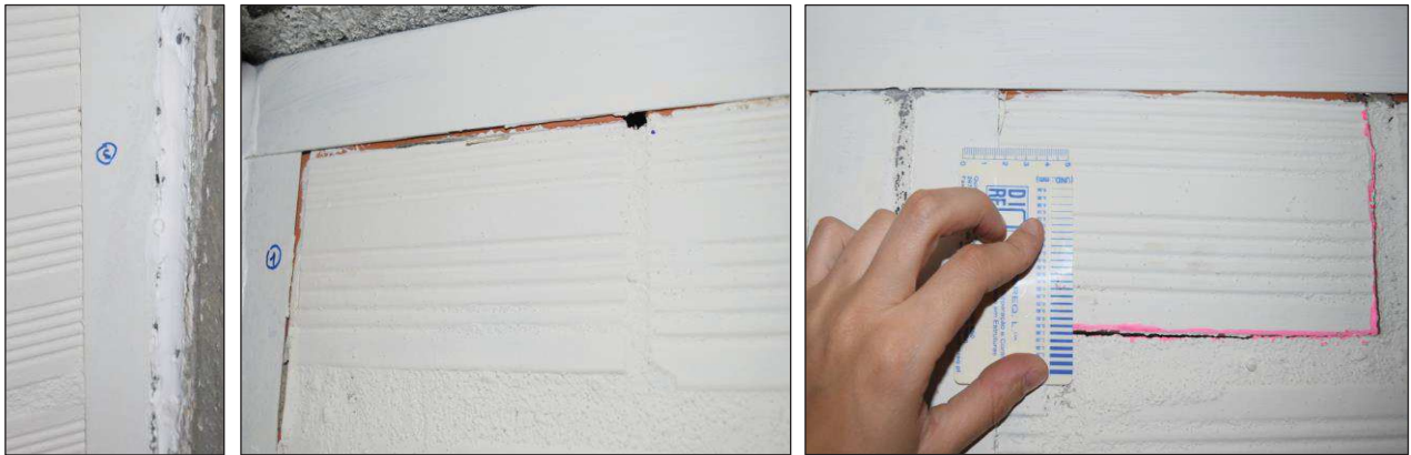
Figure 7.42. Observed damage to the low-damage masonry wall.
