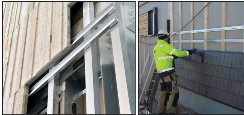
Figure 2.10. Lightweight cladding system: example of connection detail and installation of the façade (source: www.ebmsupplies.com ).
