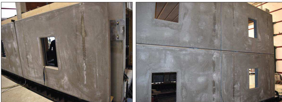
Figure D.14. Completion of the façade in the South side of the Test Building: assembly of the first level (left), final configuration of the system (right).
