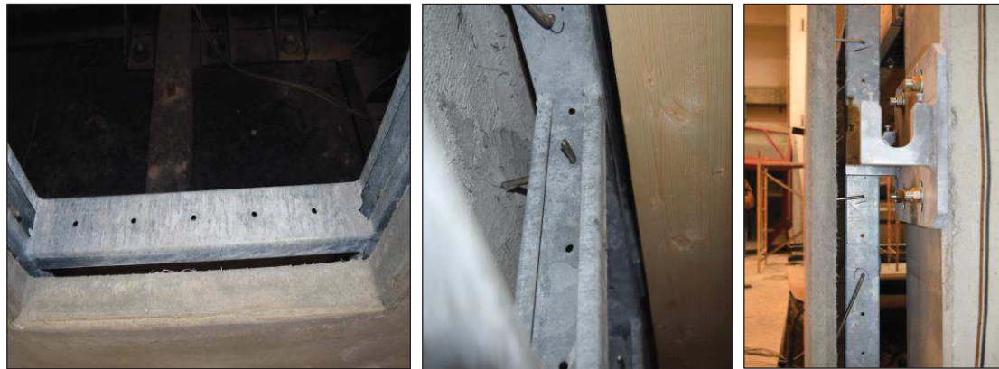
Figure D.13. Details of the GFRP panel: internal opening (left), connection of the external panel to the steel frame (centre) and sliding anchorage on the top of the system (right).
