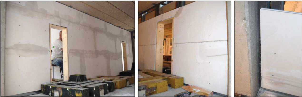
Figure 6.33. Insertion of the fiber-reinforced gypsum boards: final wall (left), first line of screws from the corners (centre) and lateral gap between wall and column (right).
