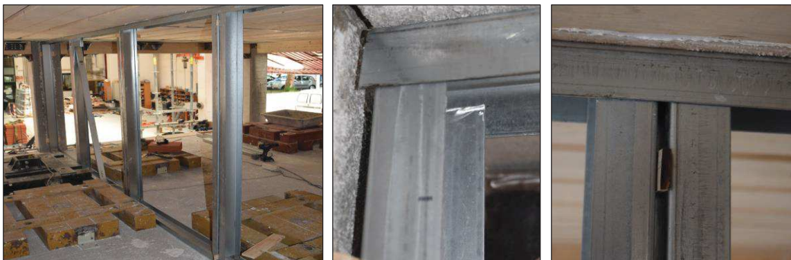
Figure 6.43. Assembly of the steel sub-frame of the masonry partition: global view (left) and detailing of the lateral (centre) and internal (right) gaps.
