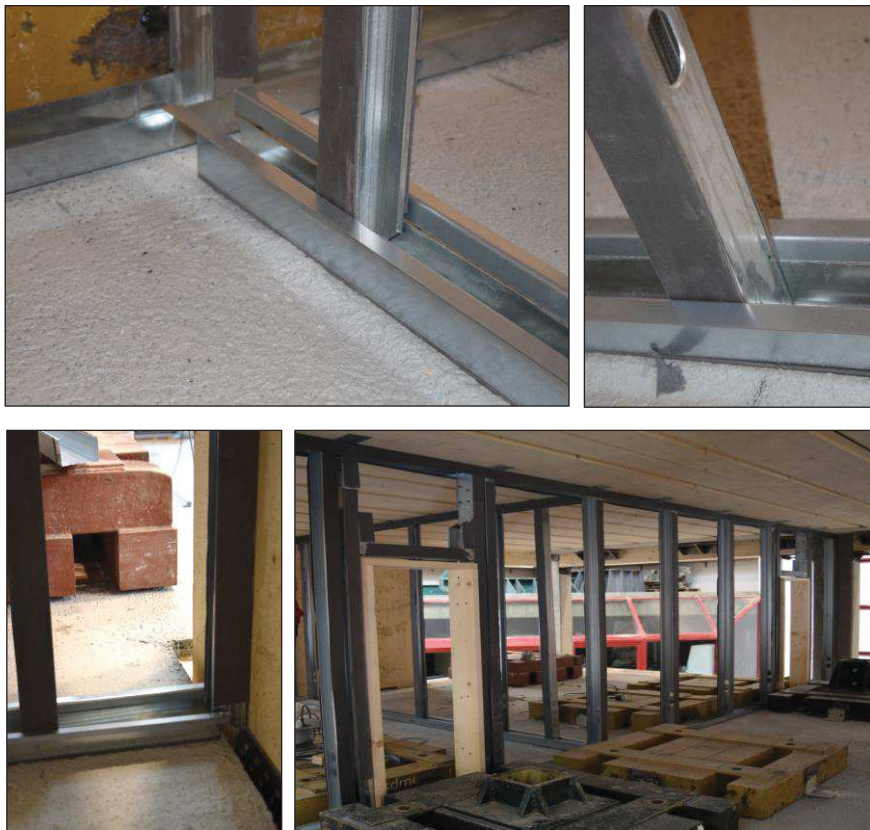
Figure D.4. Partition in the frame direction: additional L-shape profiles attached to the horizontal track on the bottom for the insertion of plants (top - left and right); detail of the connection of the horizontal track to the timber wall (bottom - left); complete assemblage of the steel frame (bottom - right).
