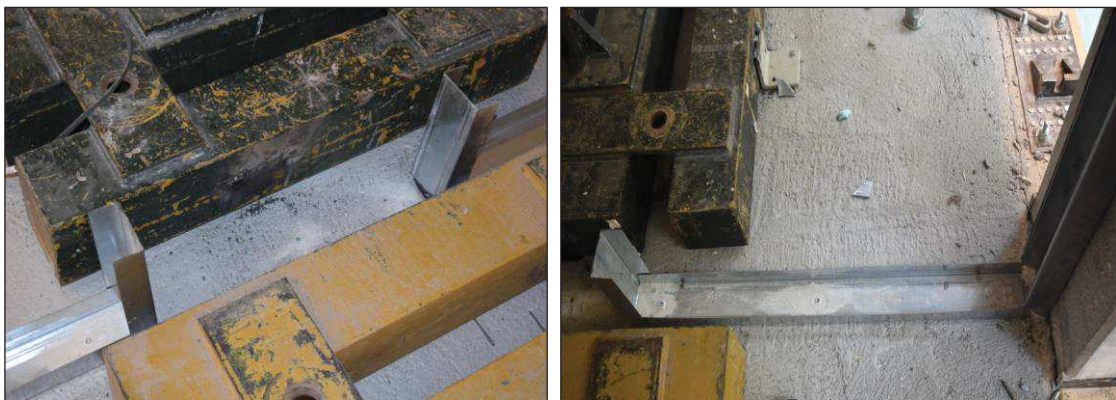
Figure D.1. Partition in the wall direction - connection of the horizontal channel of the steel sub-frame to the first floor: detail of the steel profile at the base of the opening (left) and nearby the concrete column (right).
