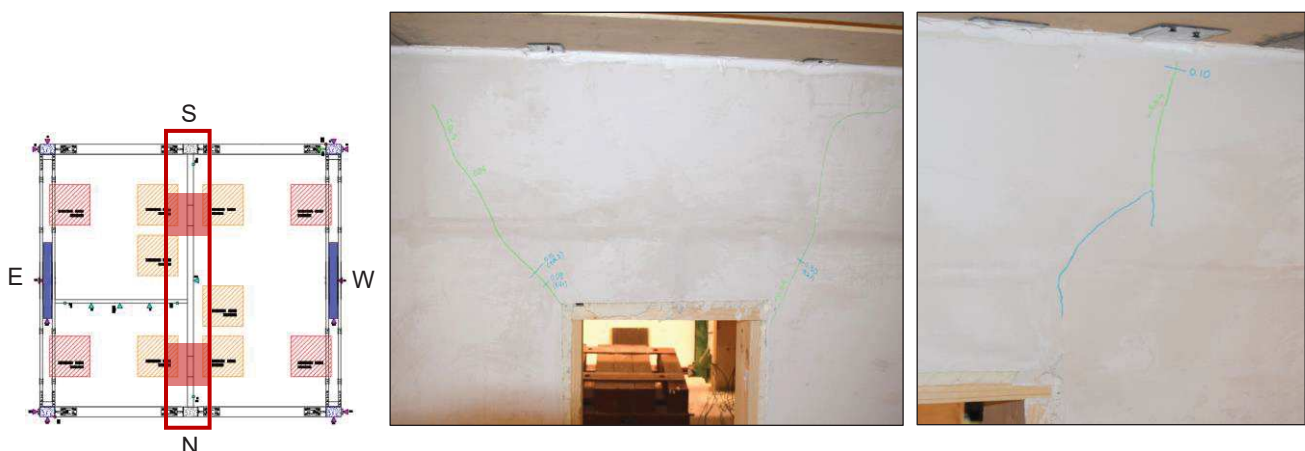
Figure 7.24. Diagonal cracks in the West side, North opening (left) and South opening (right) of the South-North wall.
