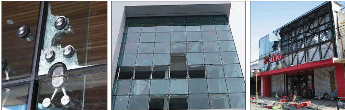
Figure 3.1. Damage to curtain walls related to broken glass (left and centre: Baird et al. 2011b; right: FEMA E-74 2011).
