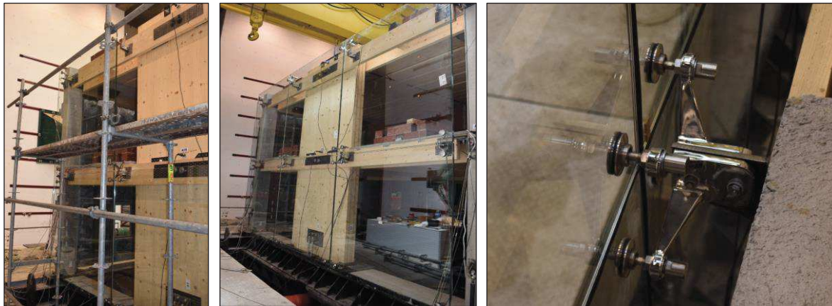
Figure D.21. Assembly of all the second level of the East-side façade: connection of the top-left panel (left), final configuration of the glass wall (centre) and particular of an internal connection system (right).
