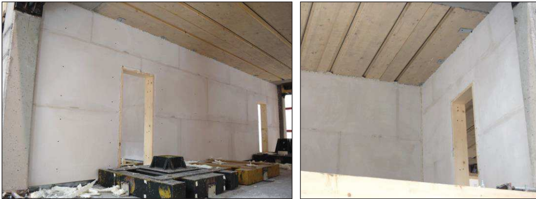
Figure D.9. Final configuration of the two partition walls in the wall (left) and in the frame (right) directions.
