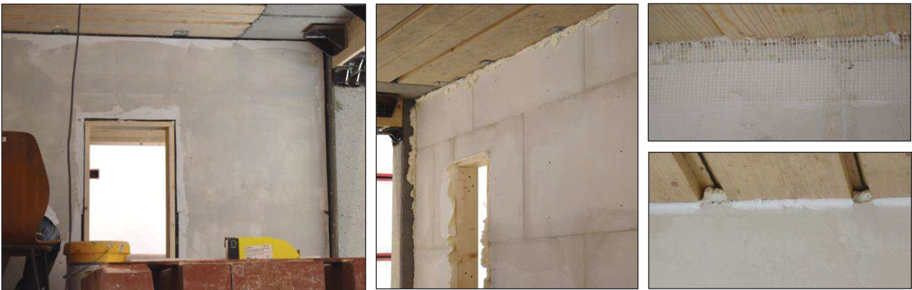
Figure 6.34. Completion of the wall: insertion of adhesive glue on the entire wall surface (left); application of silicone foam (centre); introduction of additional joint cover tape in the corners (top - right); application of silicone sealant (bottom - right).
