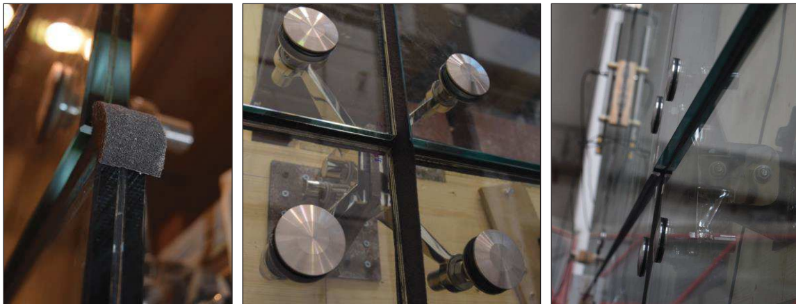
Figure 7.38. Out-of-plane movement of the panels.
