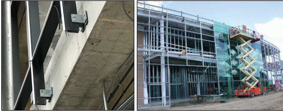
Figure 2.2. Stick curtain system: example of connection detail and installation of the façade (Eisenmann 2014).
