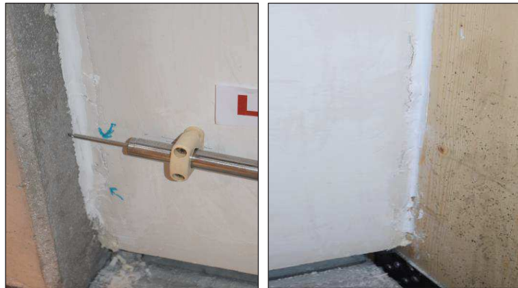
Figure 7.25. Detachment of the silicone sealant and adhesive.
