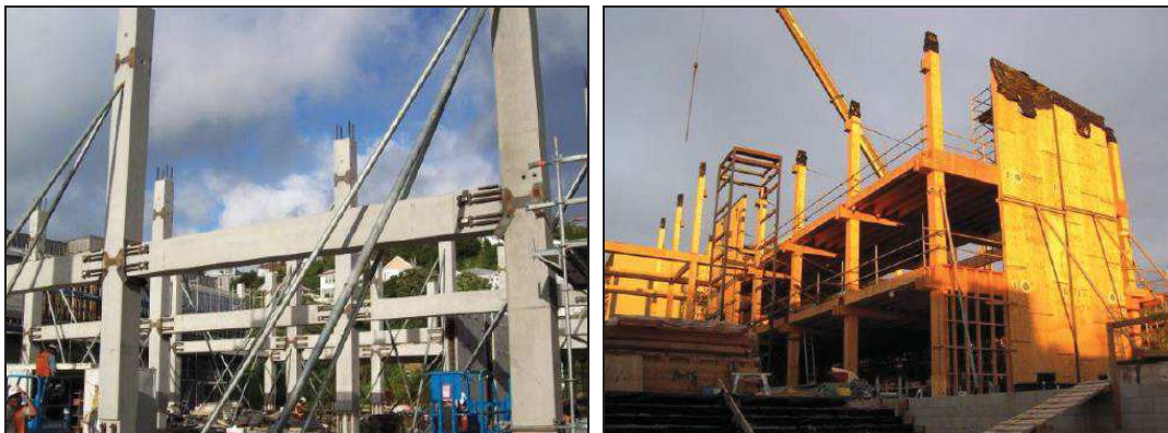
Figure 4.5. Left: Alan MacDiarmid Building at Victoria University of Wellington (New Zealand), first multi-storey PRESS building in New Zealand (Structural Engineers: Dunning Thornton Consultants; Cattanach and Pampanin 2008); Right: Nelson Marlborough Institute of Technology (New Zealand), world first Pres-Lam building (Structural Engineers: Aurecon, Devereux et al. 2011, Architects: Irving-Smith-Jack).
