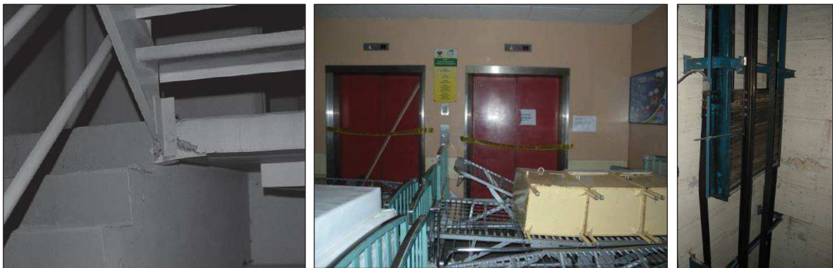
Figure 3.11. Damage to egress systems (left: Taghavi and Miranda 2004; centre and right: FEMA E-74 2011).
