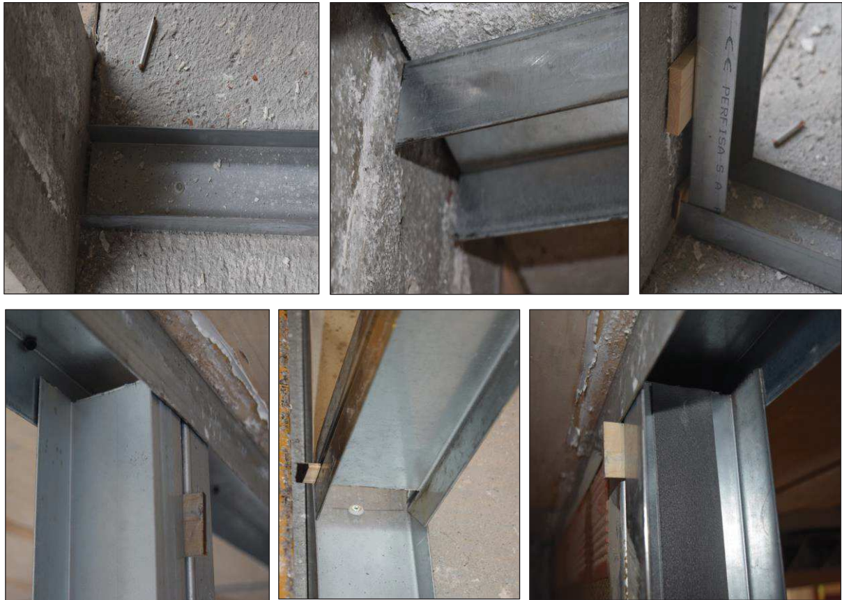
Figure D.23. Non structural detailing: gap between the column and the horizontal track on the first building level (top - left); gap between the column and the horizontal track connected to the second floor (top - centre); gap between the concrete column and the first vertical steel stud (top - right); internal gap between two vertical studs (bottom - left); detail of the bottom part of the internal steel studs (bottom - centre); introduction of an adhesive tape on the internal part of the steel profiles (bottom - right).
