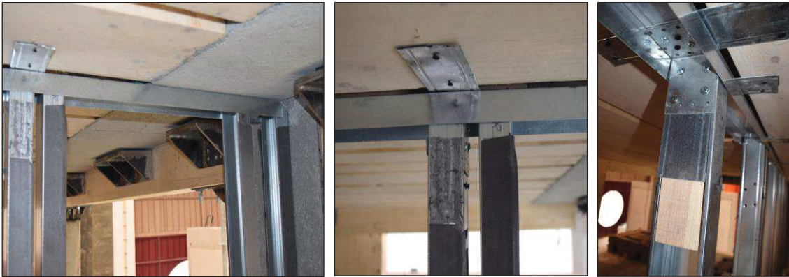
Figure D.2. Partition in the wall direction - connection of the horizontal track of the steel sub-frame to the timber-concrete beams of the second floor: view (left); additional steel pieces introduced for the connection to the timber part due to the presence of the internal hole for the wire strands (centre); telescopic joint of the steel studs of the openings connected to the upper horizontal channel (right).
