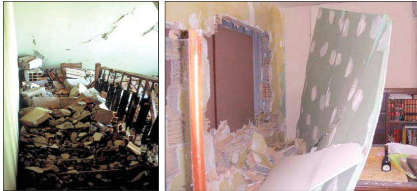
Figure 3.5. Damage to heavy partitions (left: FEMA E-74 2011; right: De Sortis et al. 2009).
