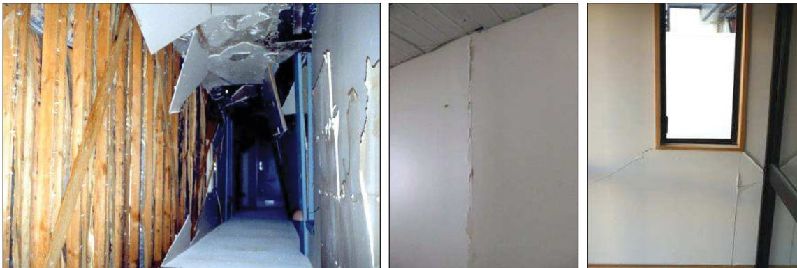
Figure 3.4. Damage to lightweight partitions (left: FEMA E-74 2011; centre and right: Tasligedik 2014)
