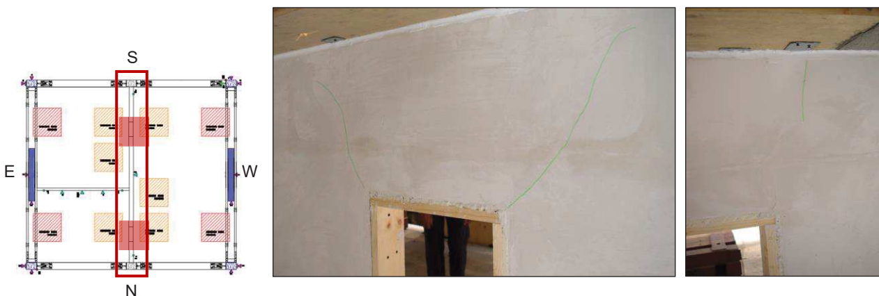
Figure 7.22. Diagonal cracks in the East side (left) and vertical crack in the West side (right) of the North opening of the South-North wall.
