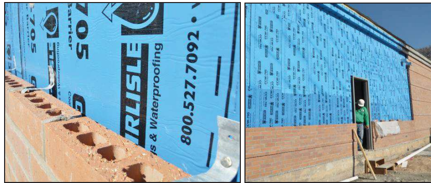
Figure 2.12. Brick veneer cladding system: example of connection detail and installation of the façade (source: www.mattrisinger.com ).
