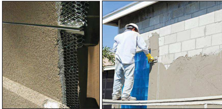
Figure 2.16. Monolithic cladding system: particular of EIFS and construction of the monolithic stucco façade (source: www.consumer.org.nz ).
