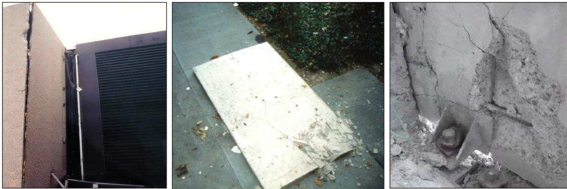
Figure 3.2. Damage to heavy precast concrete walls (left and centre: FEMA E-74 2011; right: Baird et al. 2011b).
