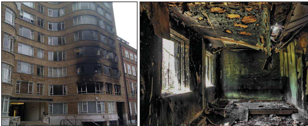
Figure 2.36. Damage to non-structural components due to fire load (source: www.wikiwand.com ).
