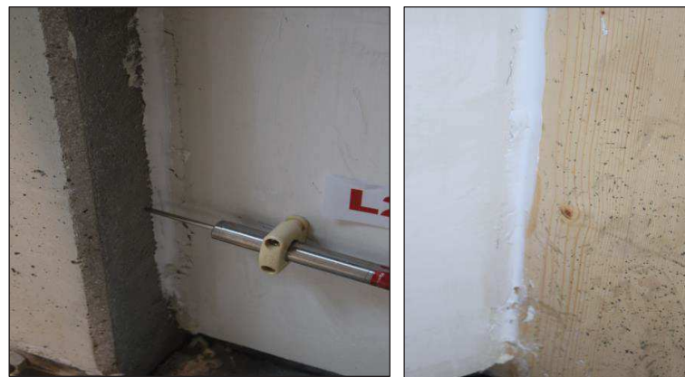
Figure 7.23. Initial detachment of the silicone sealant and adhesive.
