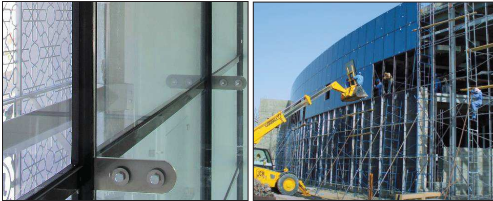
Figure 2.6. Structural glazing system: example of connection detail and installation of the façade (source: www.gip-glazing.com ).
