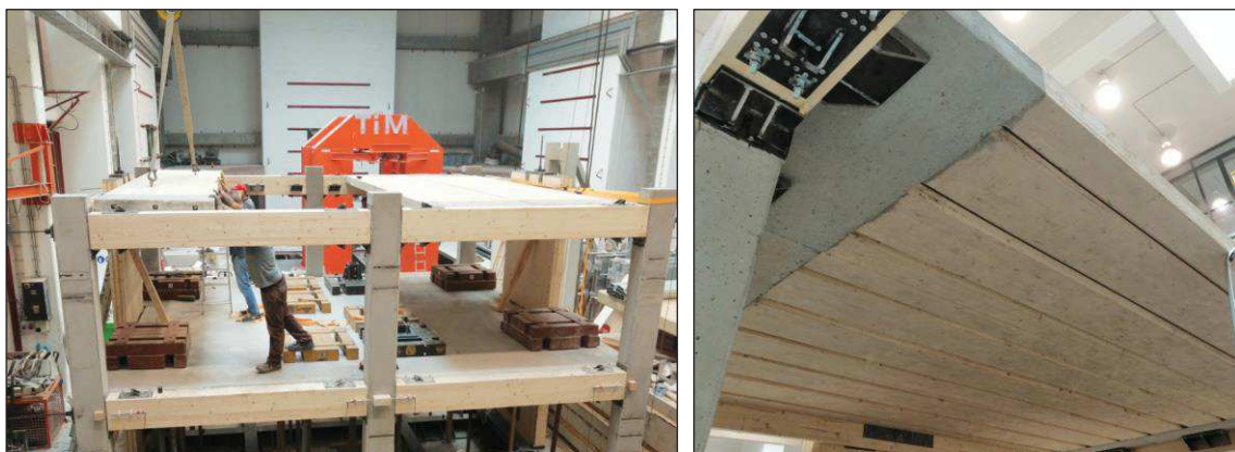
Figure 6.26. Phase 5: Lifting in place of the timber-concrete beams of the second floor (left) and final configuration of the second floor.
