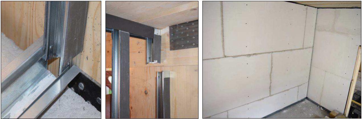
Figure 6.35. Construction of the partition wall in the frame direction: additional L-shape steel profiles (left), connection of the lateral vertical stud to the timber wall (centre), complete assembly of the panels (right).
