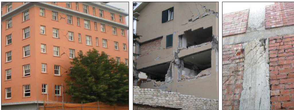
Figure 3.3. Damage to masonry infill walls (left: Baird et al. 2011b; centre: Tasligedik et al. 2011; right, Tasligedik 2014).
