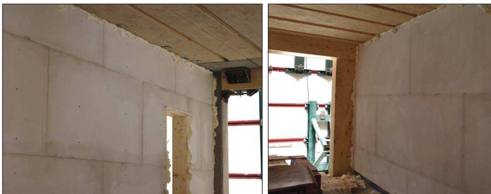
Figure D.8. Application of the sealant foam in the lateral gaps of both partition walls.
