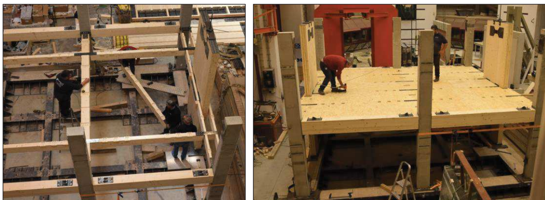
Figure 6.24. Phase 4a: Positioning of timber joists (left) and introduction of the plywood floor units (right).
