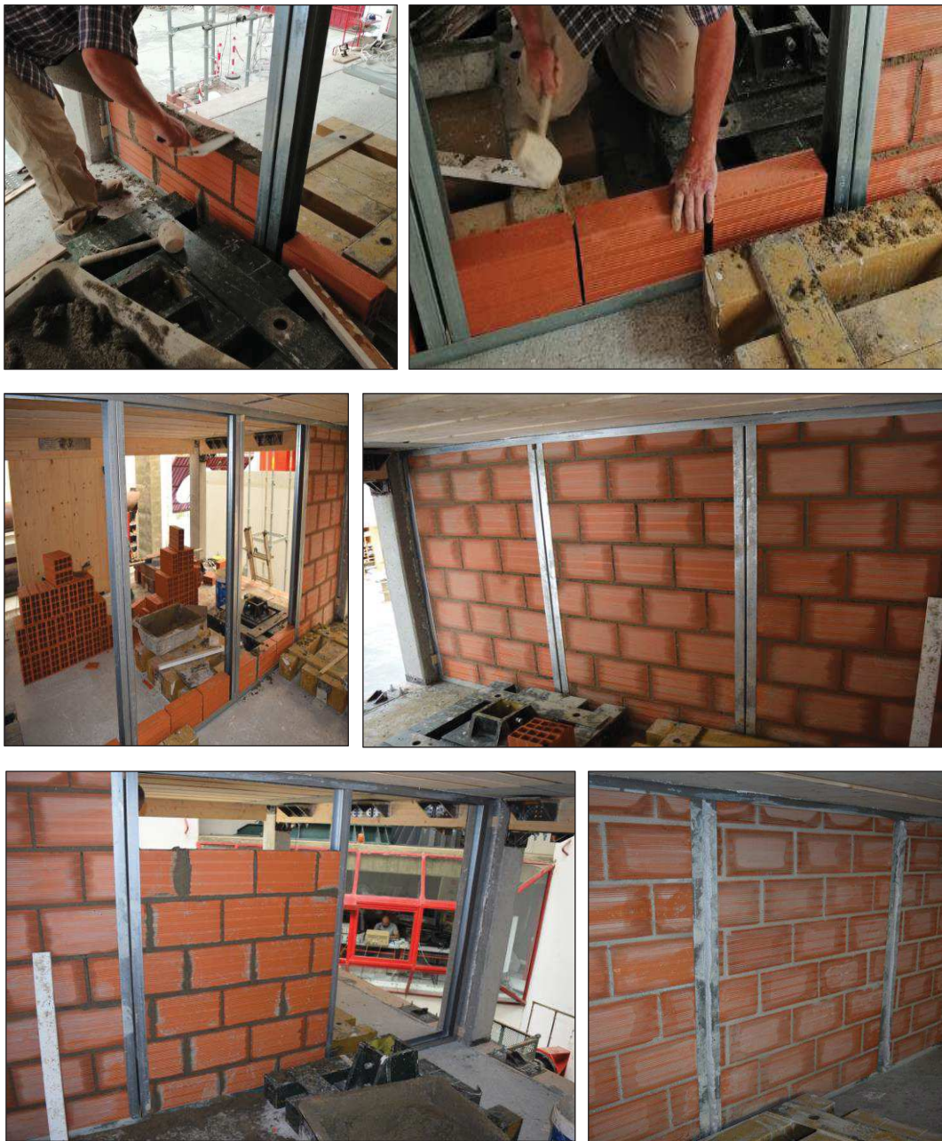
Figure D.25. Construction of the infill wall: construction of the infill panel in the North side (top - left); construction of the first brick line of the second wall from the North side (top - right); positioning of the first brick line in the central infill wall (centre - left); completion of the first three panels from the North side (centre -right); construction of the second wall from the South side (bottom - left); introduction of polyurethane foam in the lateral gaps after completing the wall (bottom - right).
