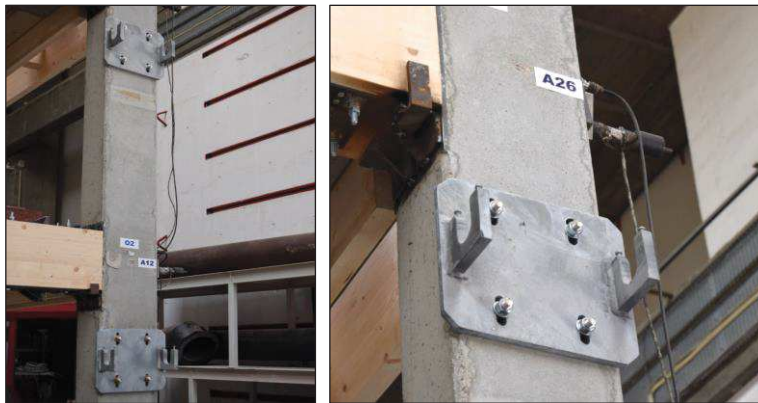
Figure D.10. Top anchorage system of the GFRC facades bolted on the concrete columns.
