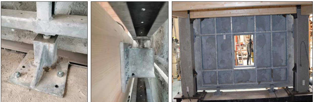
Figure 6.37. Connection of the bottom anchorages to the structural system: connection to the steel foundation (left), connection to the timber beams (centre) and internal view of a bottom panel (right).
