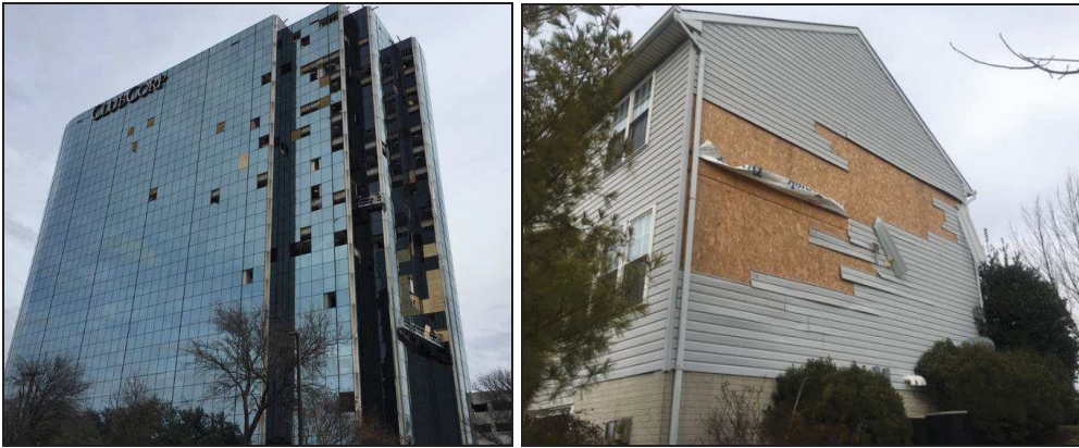
Figure 2.34. Damage to non-structural components due to wind loads (source: www.weather.gov ).
