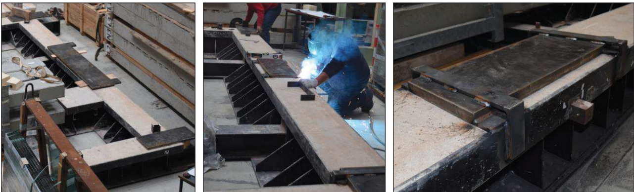
Figure 6.21. Phase 1: positioning of the steel foundation plates (left); welding of pieces of steel to fix the foundation plates to the UPN profile (centre); example (foundation plate of internal columns) of connection to the UPN profile (right).
