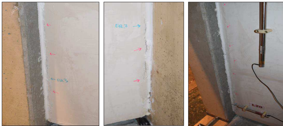
Figure 7.28. Detachment of the silicone sealant and adhesive.
