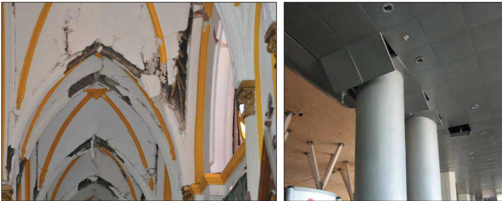
Figure 3.9. Damage to heavy ceilings (FEMA E-74 2011).
