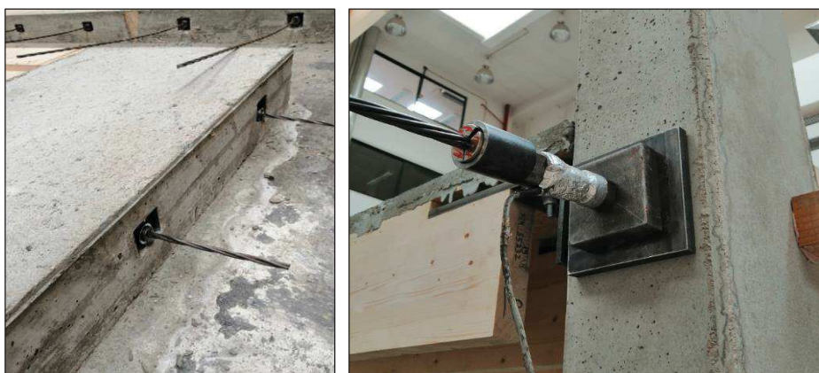
Figure 6.28. Detail of the wire-strands and anchorage system of the beams of the 3PT floor (left) and of the first-floor seismic beams (right).
