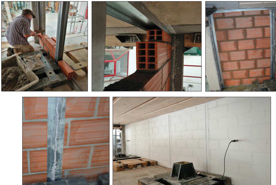
Figure 6.45. Construction of the masonry infill wall (top - left, centre) and final configuration of a panel (top - right); completion of the wall introducing polyurethane foam (bottom - left) and paint on one side (bottom - right).
