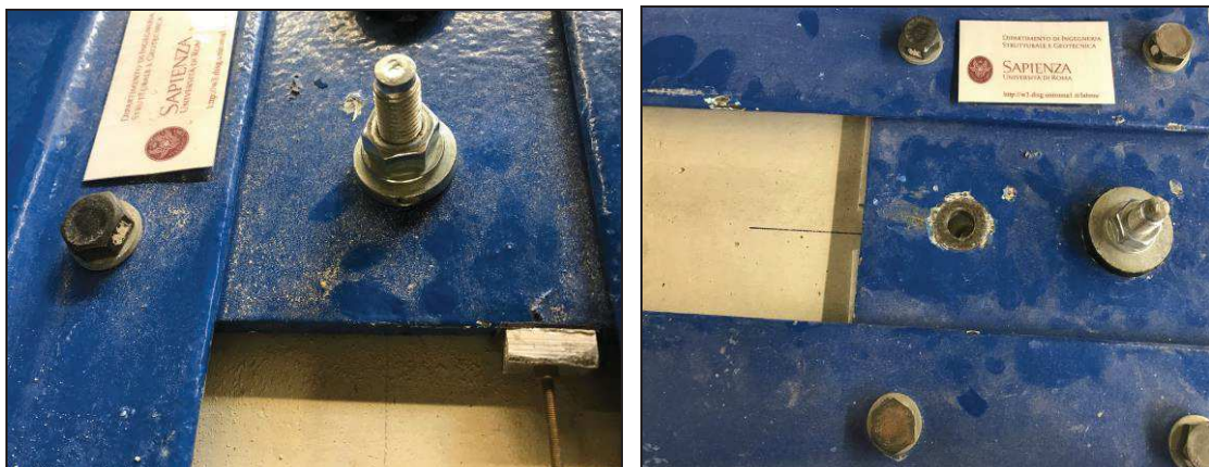
Figure A.2. Installation of the Traditional FAZ II with Mortar Filling (left) and with EQ-Rod 2.0 (right).
