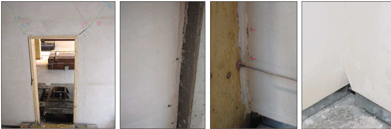
Figure 7.29. Cracking of the South-North wall in the East side, North opening (first photo) and crushing in the lateral corners of both wall partitions (other photos).
