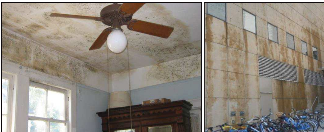
Figure 2.38. Damage to non-structural components due to weather tightness (source: www.vitorealizza.com ).
