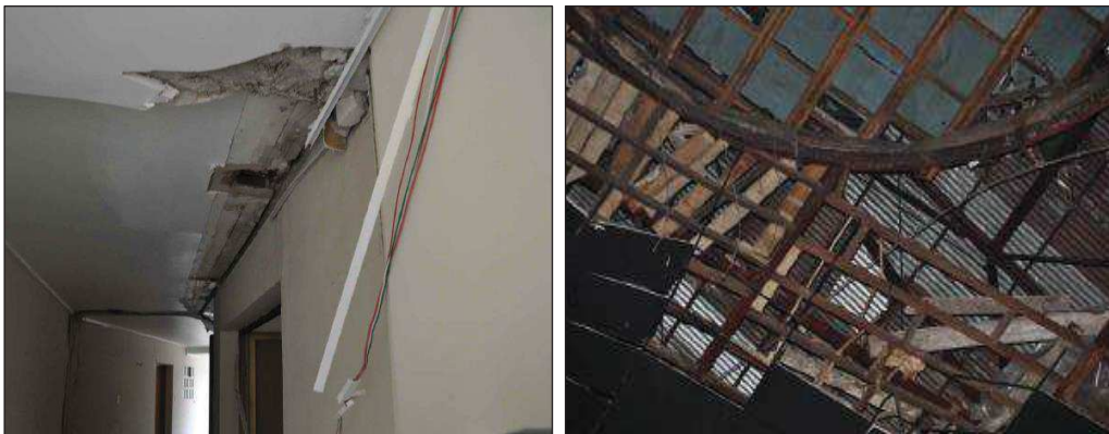
Figure 3.8. Damage to ceilings adherent to the building floors (FEMA E-74 2011).
