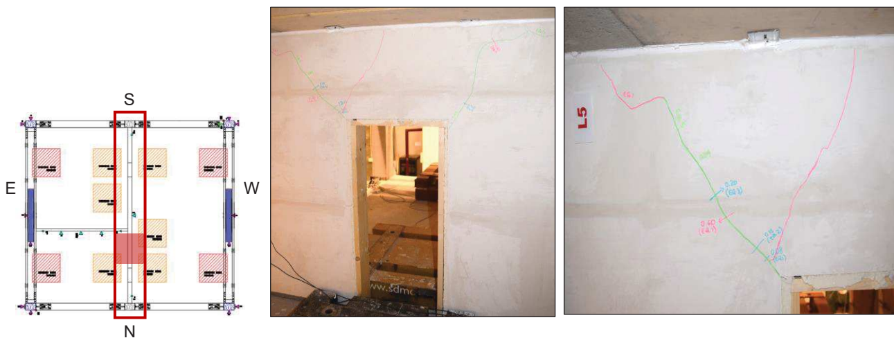
Figure 7.26. Cracking of the South-North wall in the West side, North opening.
