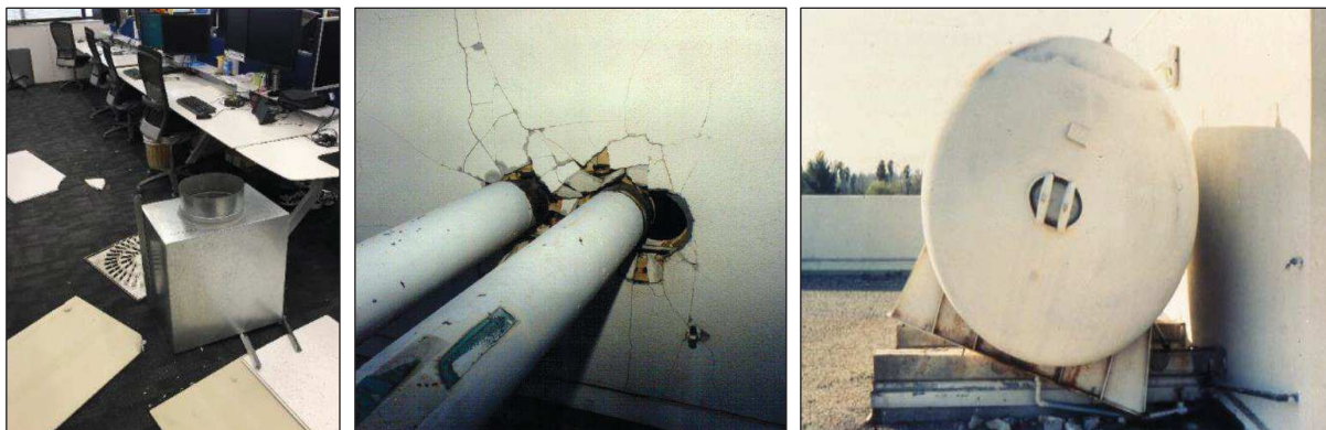
Figure 3.10. Damage to building services (left: Baird and Ferner 2017; centre and right: FEMA E-74 2011).
