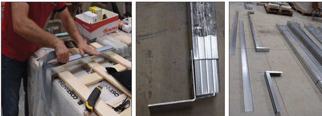
Figure 6.30. Steel frame construction: application of the adhesive (left); telescopic (slip) joint (centre); horizontal guides with the vertical extension forming base of the door frame (right).
