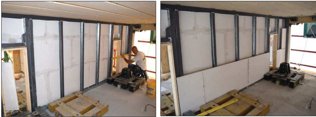
Figure D.6. Partition in the wall direction - realization of the gypsum wall connecting the ceramic panels through their male-female joints and adding adhesive glue between the panels.
