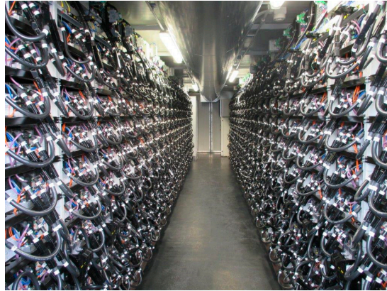
Figure 2. Racks for battery strings, installed inside an air-conditioned cabinet.
