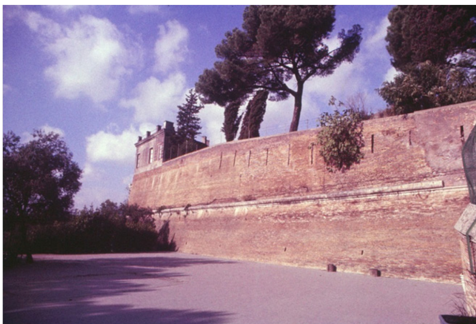
Fig. 20. General view of the masonry, highlighting the toro and the loopholes. Photo by C.B. 1985.
