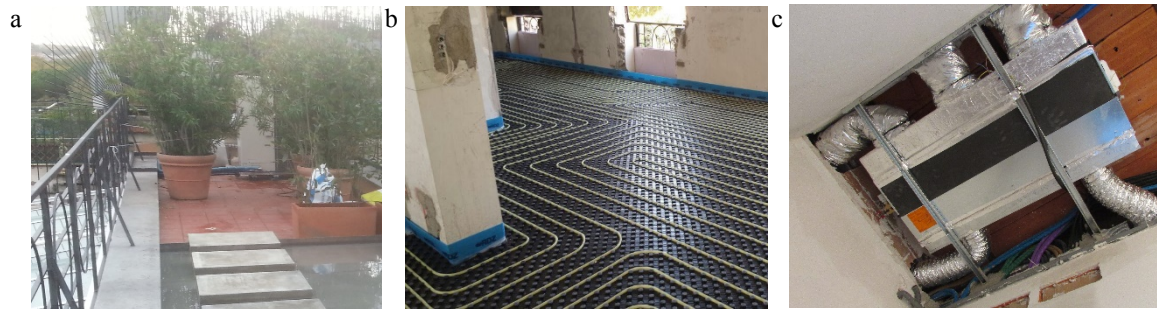
Fig. 3. Heating and cooling systems (a) Heat pump; (b) Radiant floor panels; (c) Ducted fan coils.
