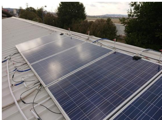
Fig. 1. General view of the PV panels.
