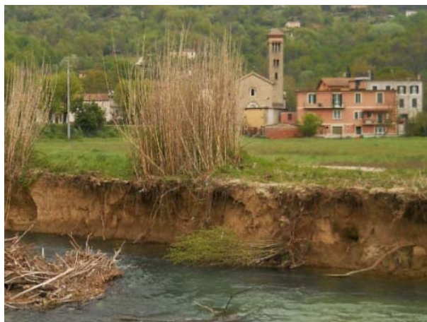
Fig. 11 A current picture of a needed bank protection intervention
