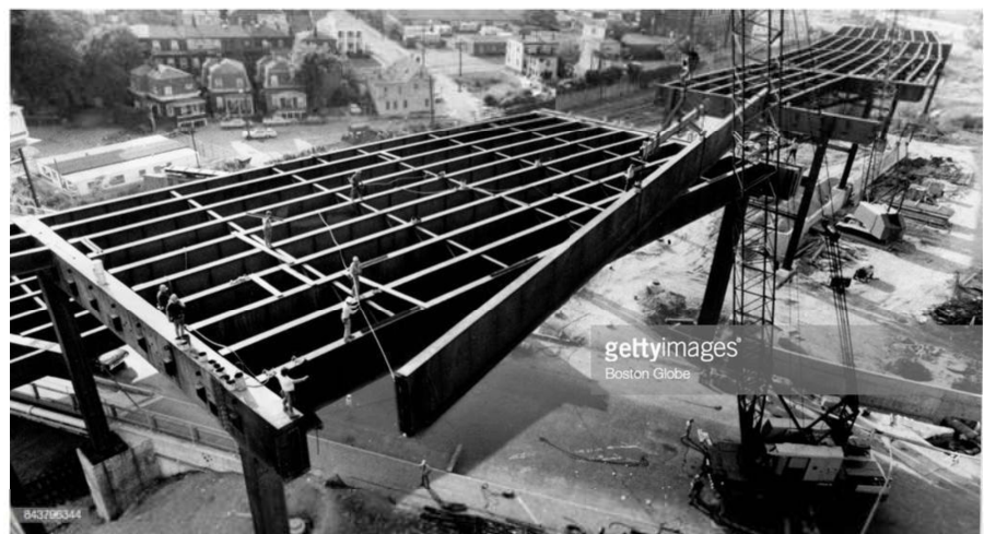
Fig. 4 - The construction of the Interstate 93, June 13, 1971, Photo by Ellis Herwig, The Boston Globe via Getty Images
