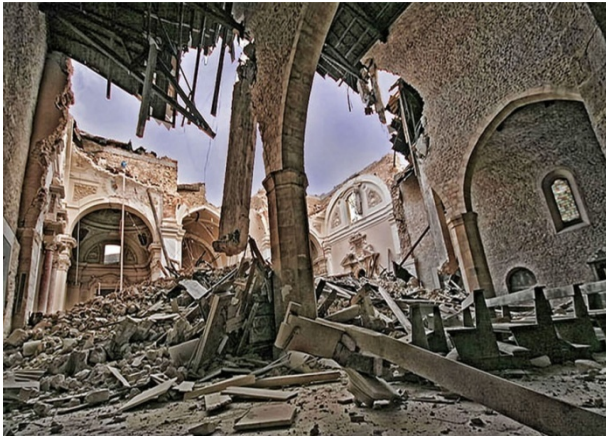
Fig. 6 April 6th, 2009: the collapse of the dome.
