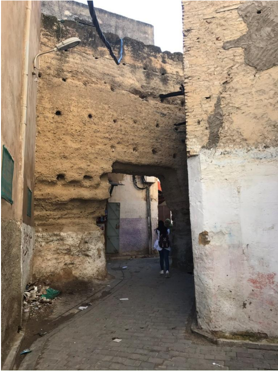
Fig. 5: A damaged earthen structure of the Milla (Jewish) district.
