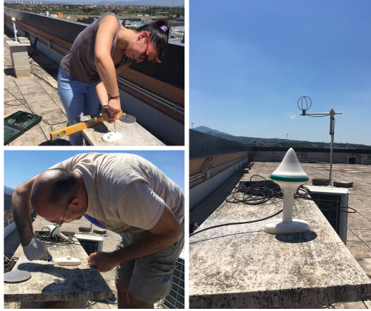
Fig. 3.3: LOW2 Single-frequency receiver installation
