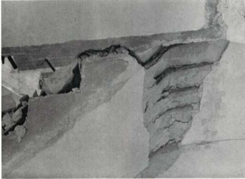
Figure 2.13: Irpinia earthquake (1981), detachment between the staircase flight and half pace.
