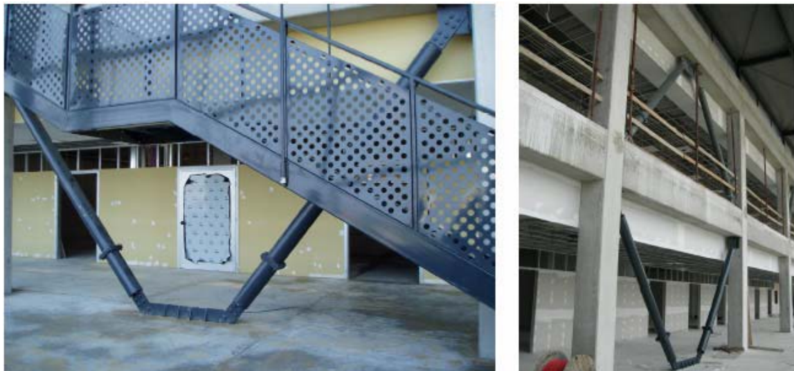
Figure 3.14: Two BRBs installed in the new building of the university of Ancona
