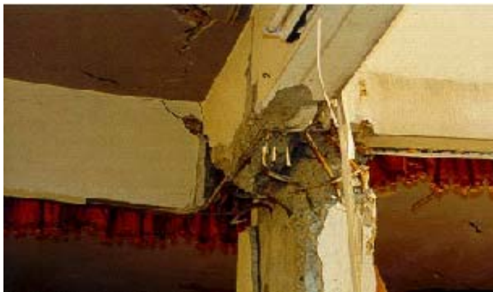
Figure 2.19: Kobe earthquake (1995), beam-to-column joint failure.
