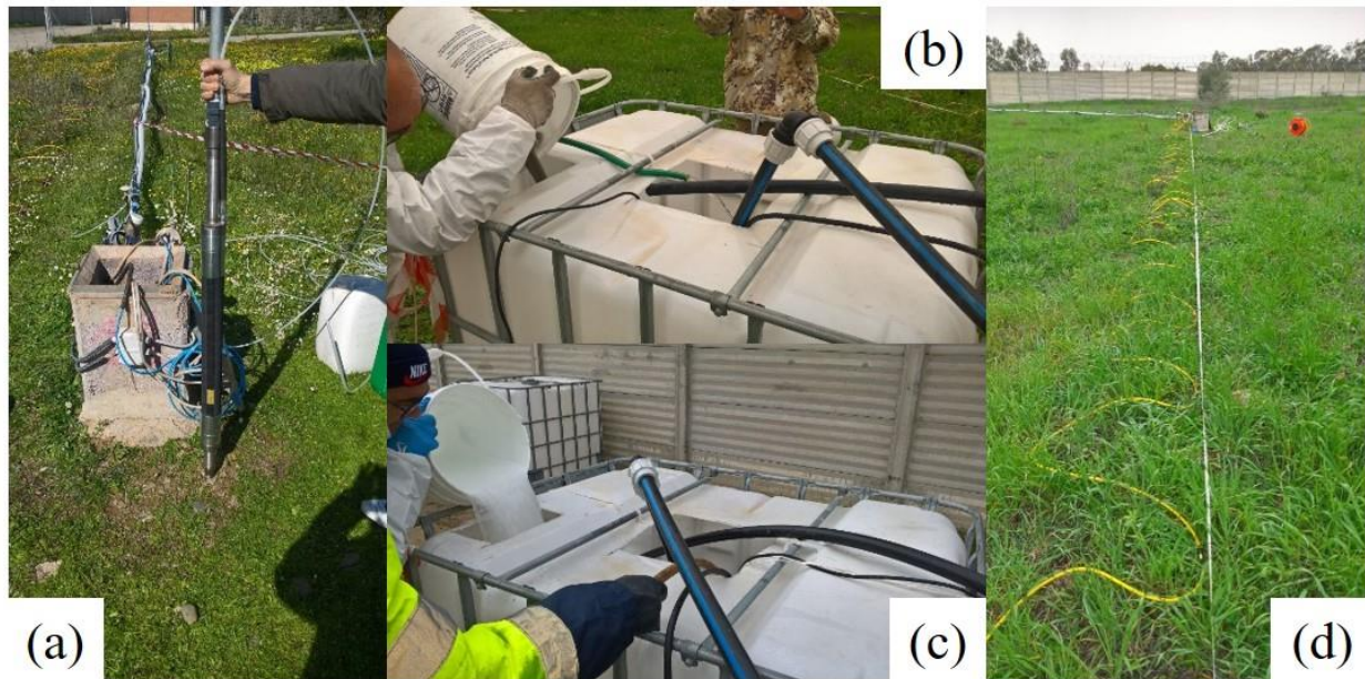
Figure 12. Pump used for the injection of different reagents in groundwater (a, b, c), ERT line realized in conjunction with the injection of amendments.
