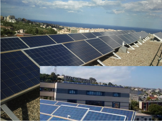
Figure 6: An overview of the PV plant at the campus.
