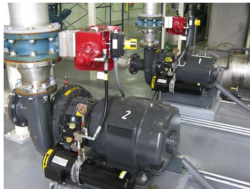
Fig. 9. Rentricity flow-to-wire installation, Keene, NH.
