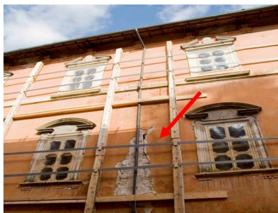
Figure 2. Historical Library of the University of L'Aquila (Italy) damaged for the earthquake (photo Prof. F.Bontempi).
