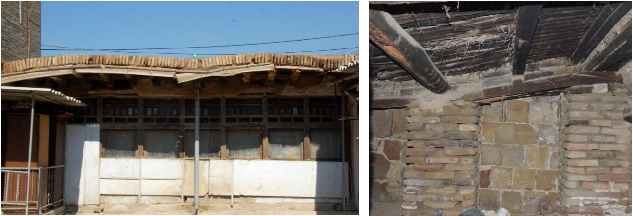
Figure 3.33 Deformation of the ceiling because of high pressure on the roof; Tehrani House, NW building mass. Figure 3.34 Extreme inclination of the ground level due to flooring heaviness of the upper story, Nili House.
