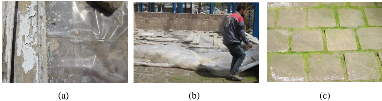
Figure 4.8 (a) moisture retention on the roof of the northwestern mass due to the use of plastic as a protective cover, (b) removal of plastic cover, (c) weeds growth between brick rows. (Govahi 2015)
