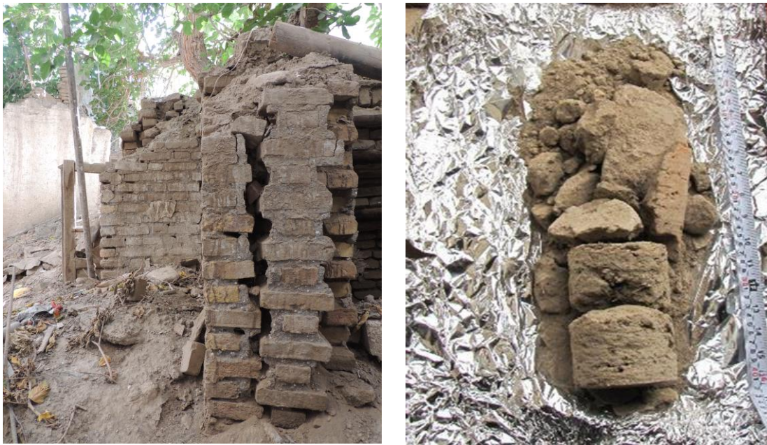
Figure 3.23 Splitting of burnt-brick masonry in the north-earthen quarter of Nili House. Figure 3.24 The sun-dried brick rubbles found from the central part of masonry in the western building mass of Darugheh House. (Govahi, 2012)
