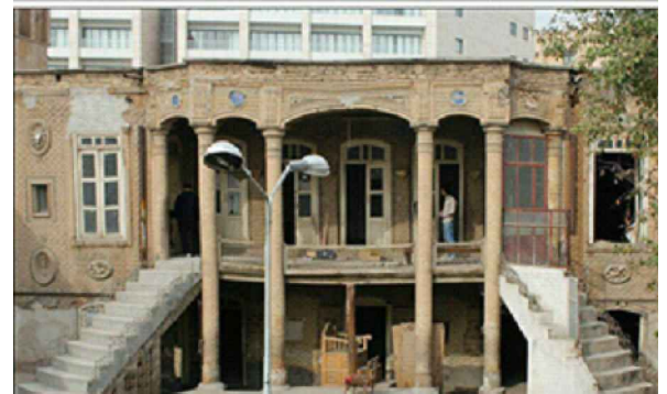
Fig. 4.12.1 Deformation of the balcony in the northwest building mass.
