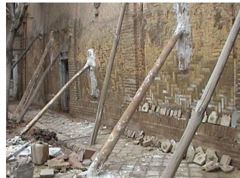
Fig. 4.2.2 Inappropriate connection between wooden props and the brick wall using gypsum mortar to paste.
