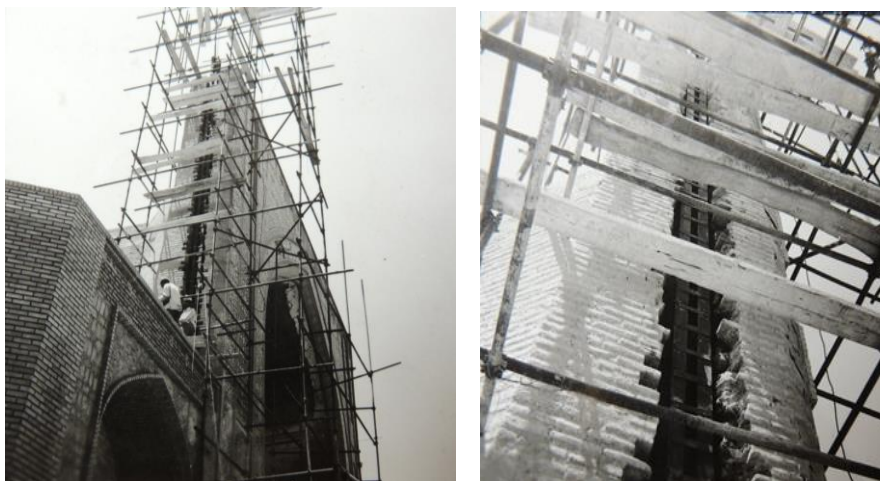
Figure 4.13 Implementation of steel structure in consolidation of Paien Khiyaban’s Mosalla, 1973; insertion of steel column in the brick masonry.
