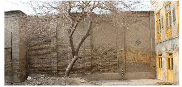
Fig. 4.6.1 Physical condition of southwestern boundary wall before the onset of restoration operation.
