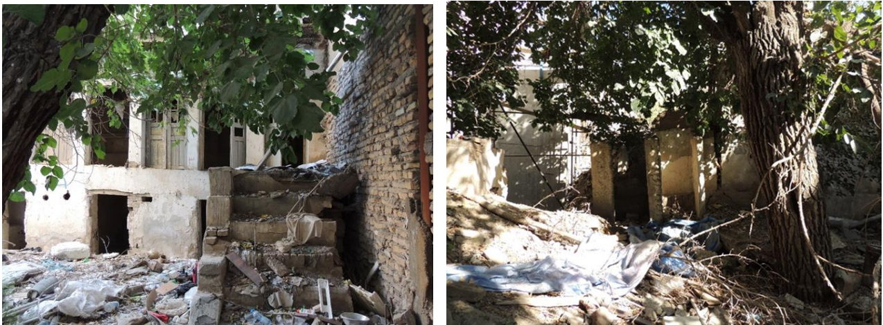
Figure 2.45 Construction of staircase in the courtyard in order to create separated entry into the western rooms on the first floor, southwestern mass. Figure 2.46 The new walls built on the eastern side of courtyard to make new spaces like bathroom.
