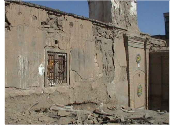
Fig. 4.4.1 Physical condition of southwestern wall before the onset of restoration operation
