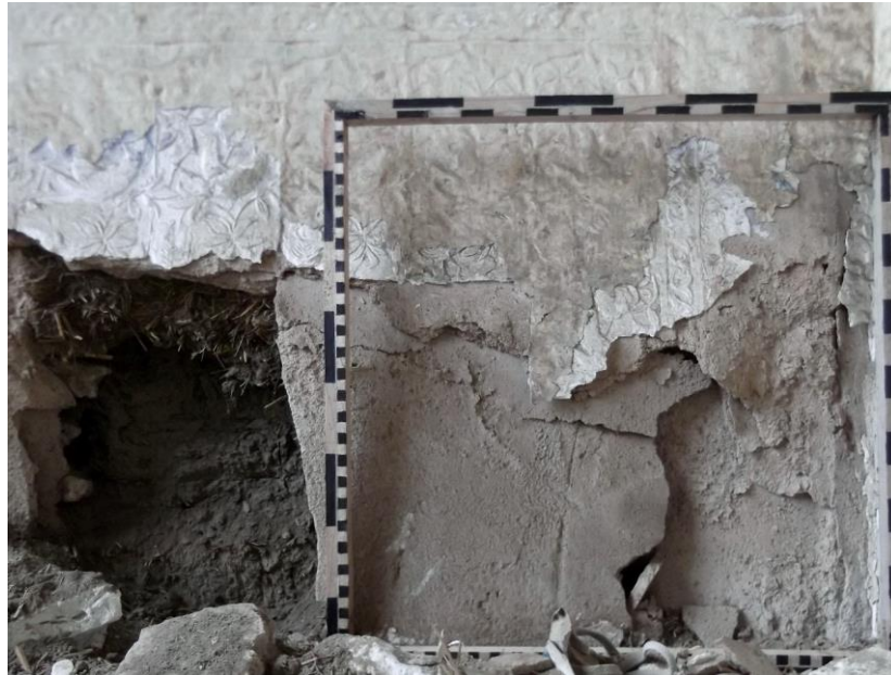
Figure 3.28 The blistering and delamination of mud-gypsum plaster layers caused by expansion of the humidity.
