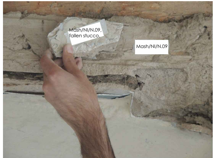
Nili's house, first floor, guest room, northeastern wall, Mash/NI/N.09, fallen stucco.
