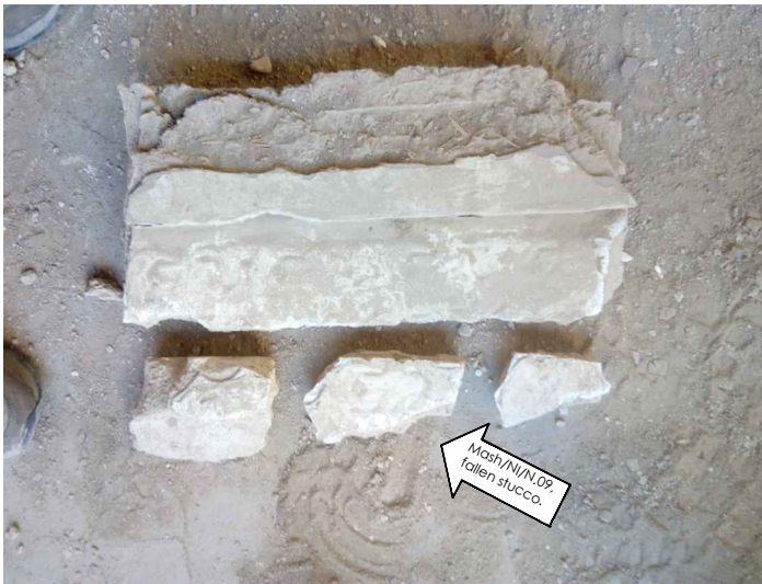
Nili's house, first floor, guest room, fallen decorative stuccoes.
