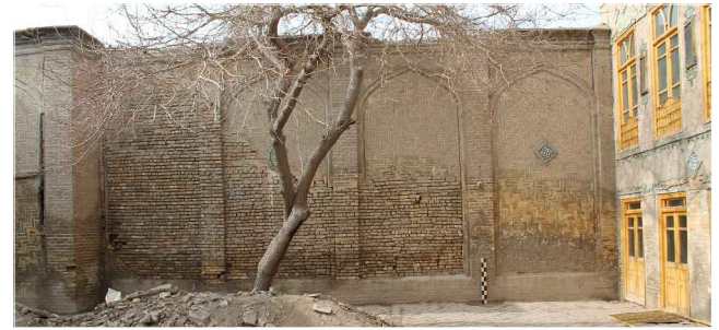
Fig. 4.8.1 Physical condition of southwestern boundary wall before the onset of restoration operation.
