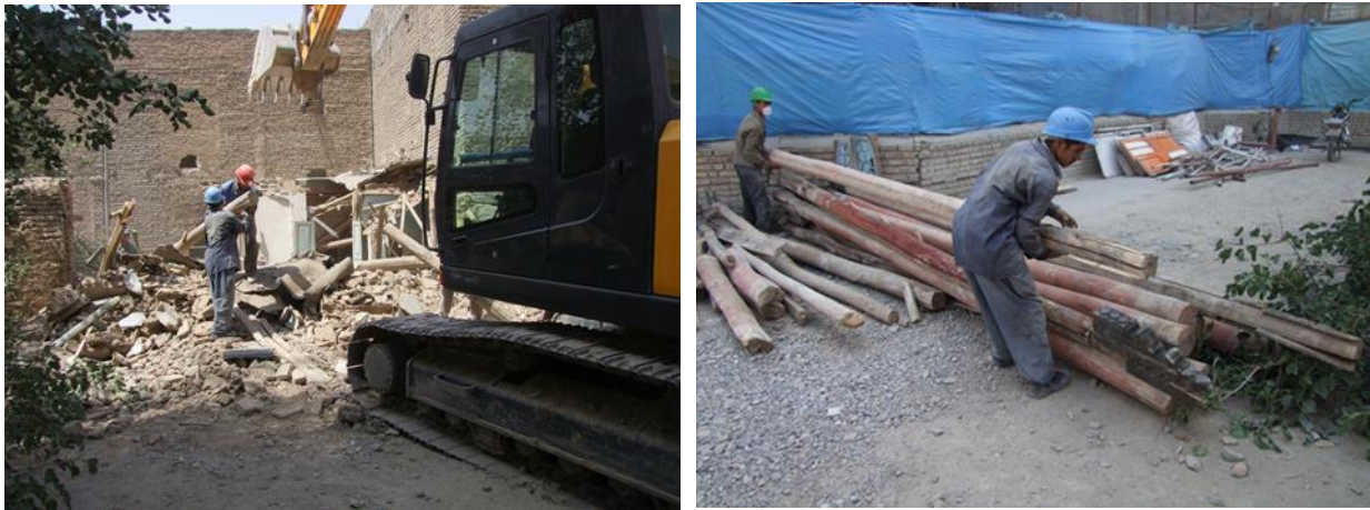
Figure 4.11 Collecting the materials during the demolition of a traditional house in Mashhad. (Govahi 2013)
