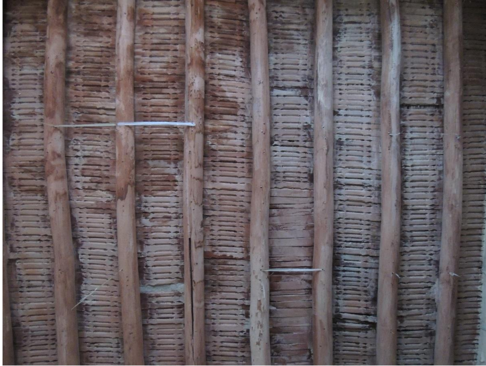
Figure 3.31 The combination of round beams and wooden planks in timber ceiling of living room in Nili House.
