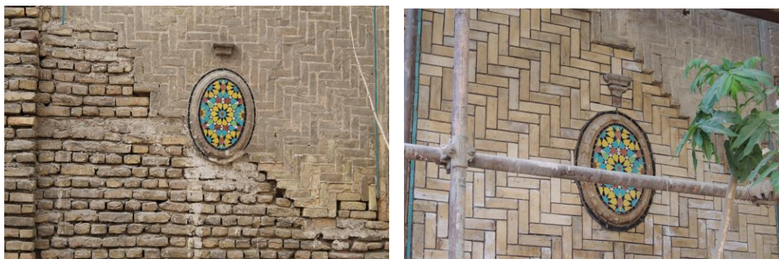
Figure 4.10 Sottosquadro method; leaving evidences between the restored and original portion of southwestern boundary wall, original (above) and restoration (below).
