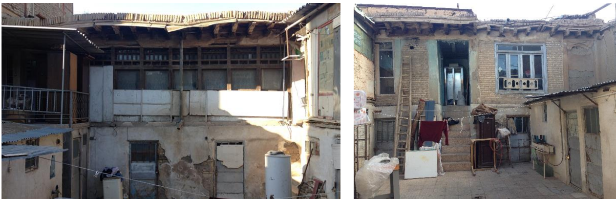
Figure 2.49 The current state of the summer quarter façade, northwestern mass. Figure 2.50 The winter quarter façade, southeastern building mass.
