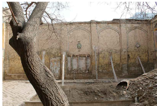
Fig. 4.2.1 Use of wooden props and beams to prevent the collapse of the northeastern boundary wall.
