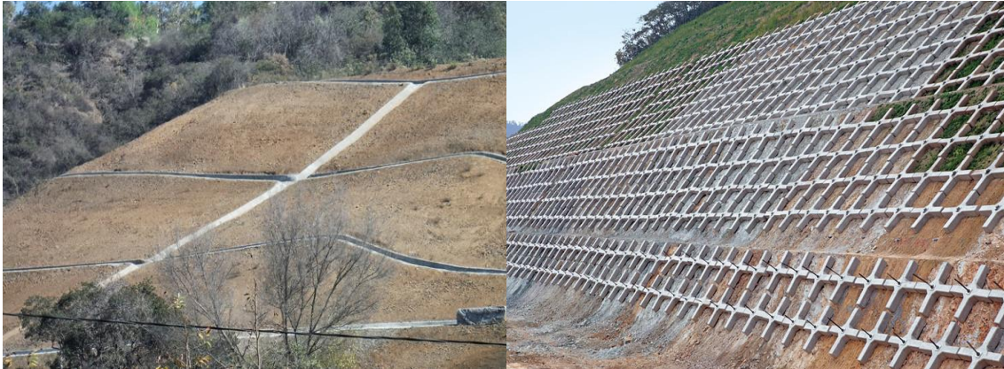
Figure 4 - Drainage system (left) and anchorage grid (right) (sources: Weinstein Construction Corp and Dywidag systems)
