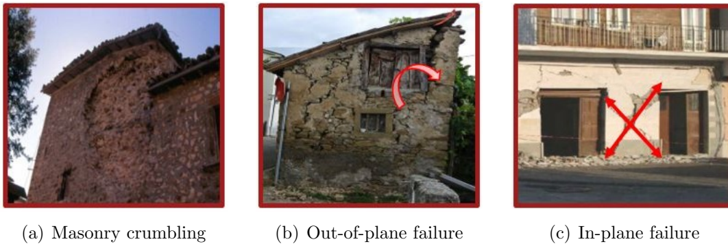
Figure 1.3: Failure mechanisms of masonry structures.
