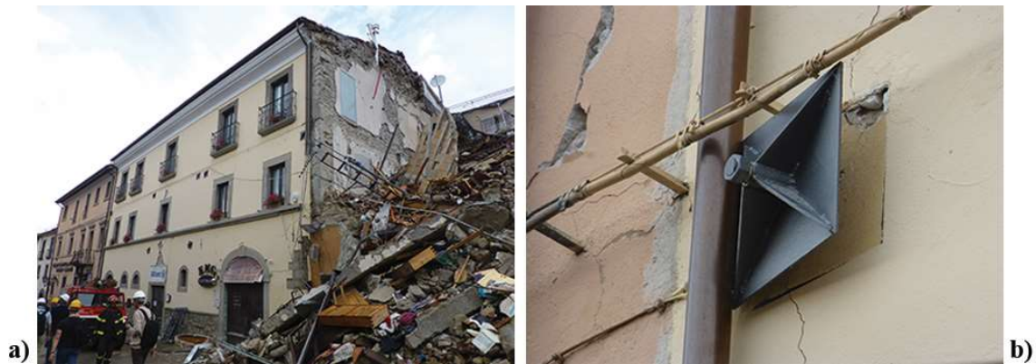
Figure 1. Amatrice, Central Italy. a) Building strengthened by steel tie rods survived the 2016 earthquake, whereas nearby one collapsed, b) close up of wall anchor and permanent displacement of tie rod.
