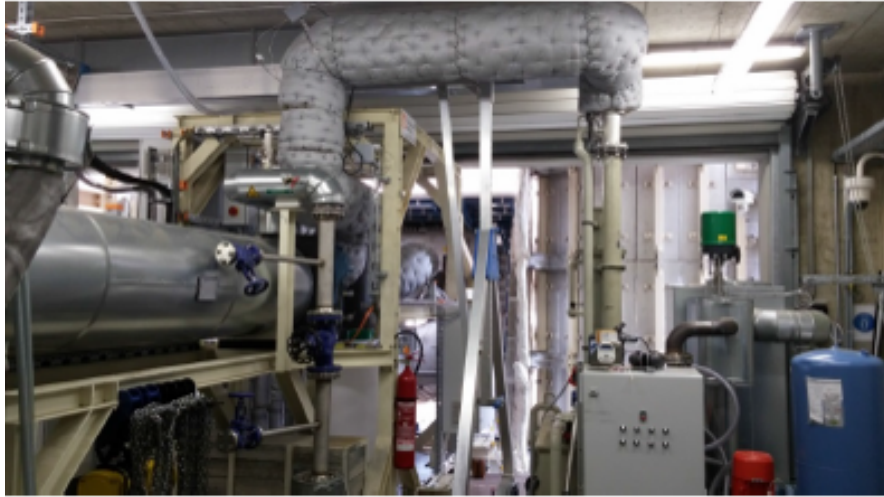
Figure 6.3: Picture of set up DEMO plant. Reference: Thomey et al. [2016]
