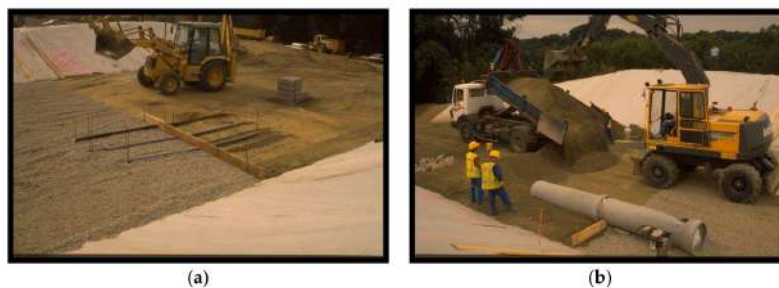
Figure 12. Placement of (a) one of the pipe series in the gneiss sections, and (b) the 500-mm concrete pipe.
