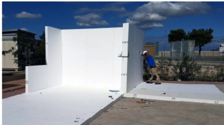
Figure 2. From residential emergency, fixed in time, to an eco-sustainable/environment-friendly solidarity architecture dilated in time in order to the interpretation of the new demand, photo AC Engineering
