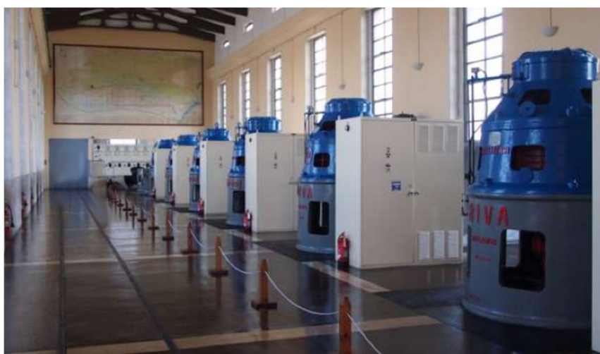
Figure 2. Hydraulic pumps in Mazzocchio's pumping station.
