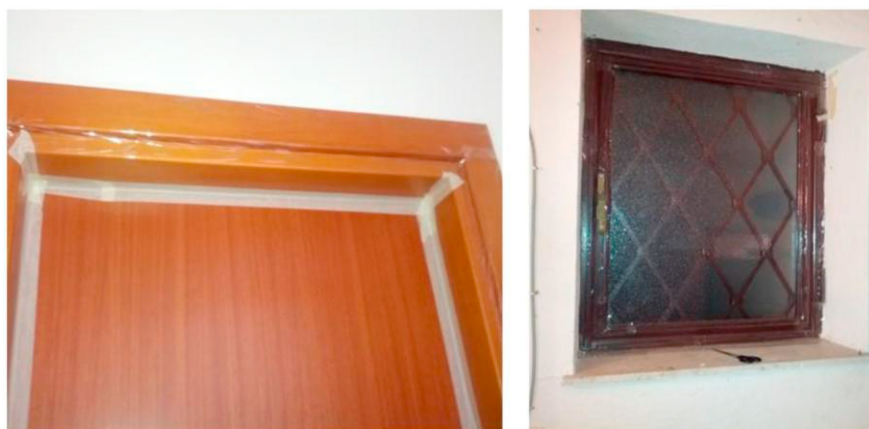
Figure 2 – Doors and windows sealing by plastic and paper scotch, simulating air-tight doors and windows.
